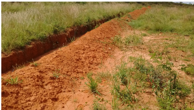
FIGURE 1 Trench for rainwater harvesting to enhance native pasture production and revegetation (Photo credit: Kevin Z. Mganga).
