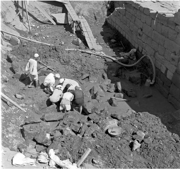
Figure 17. Chevrier's 1940s excavation in front of the western tribune. The two mooring rope loops in course four and five are visible. The pump is located at c.70.50 m, five masonry courses below the stone loops (Photo no. 6112 ©CFEETK).
