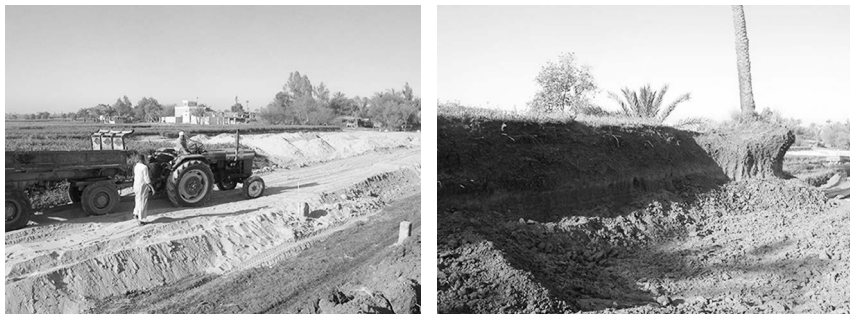
Figure 3. Wadi material is being used to level former Nile channels (left), whereas the banks of the former channels are being bulldozed (right) and the excavated Nile silts are being used as topsoil in the infilled channels. Pictures are taken 2 km south of Dayr al Barshā.
