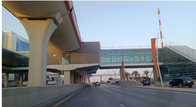
Figure 6. The Riyadh Metro project: Work in progress, pedestrian bridge for the metro station.
