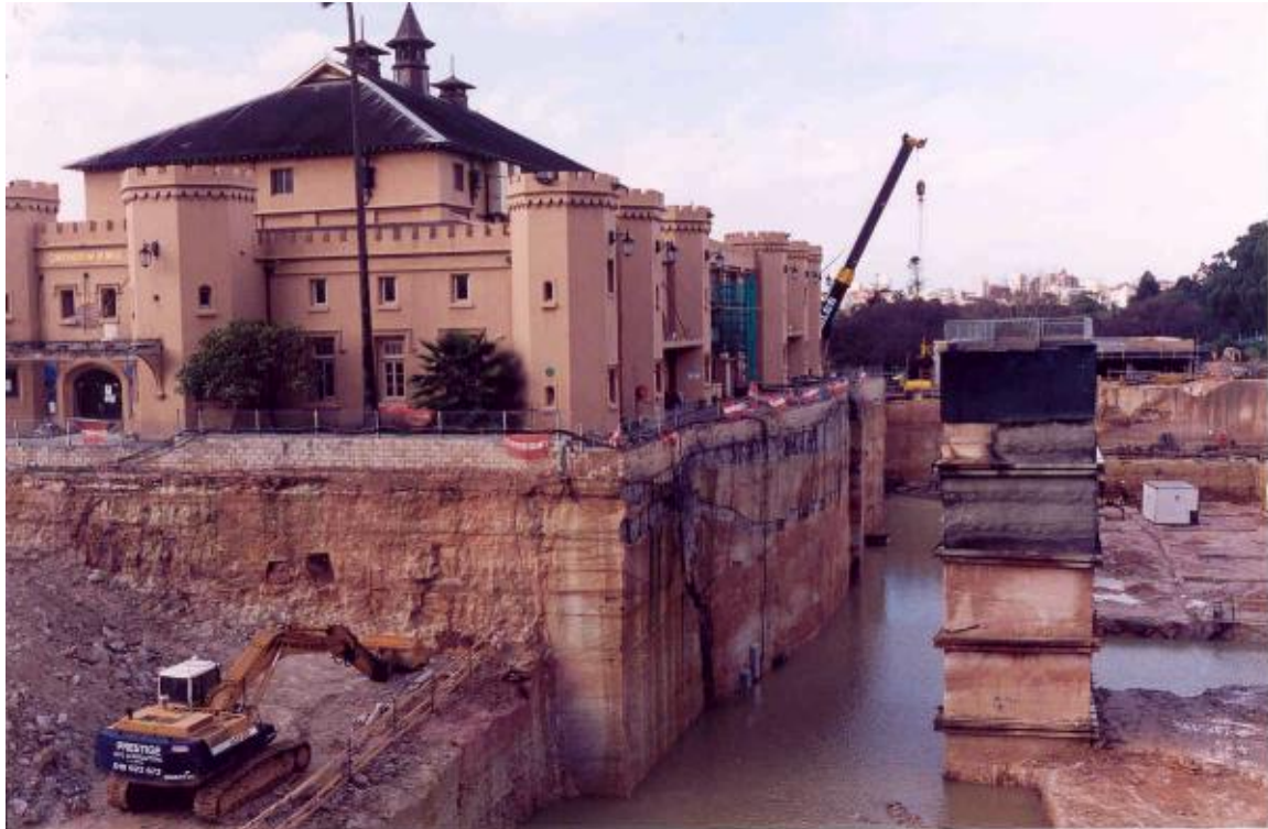
Figure 4.4: The pillar of rock on the right-hand side of the image is supporting an area of in situ archaeological remains that would eventually become one of the key archaeological displays inside the main foyer of the new underground extension of the Sydney Conservatorium of Music. This presented a logistical and engineering challenge, which significantly increased the construction costs. It was one of five areas of in situ archaeological remains retained within the new building (Image Credit: Caitlin Allen 1999).
