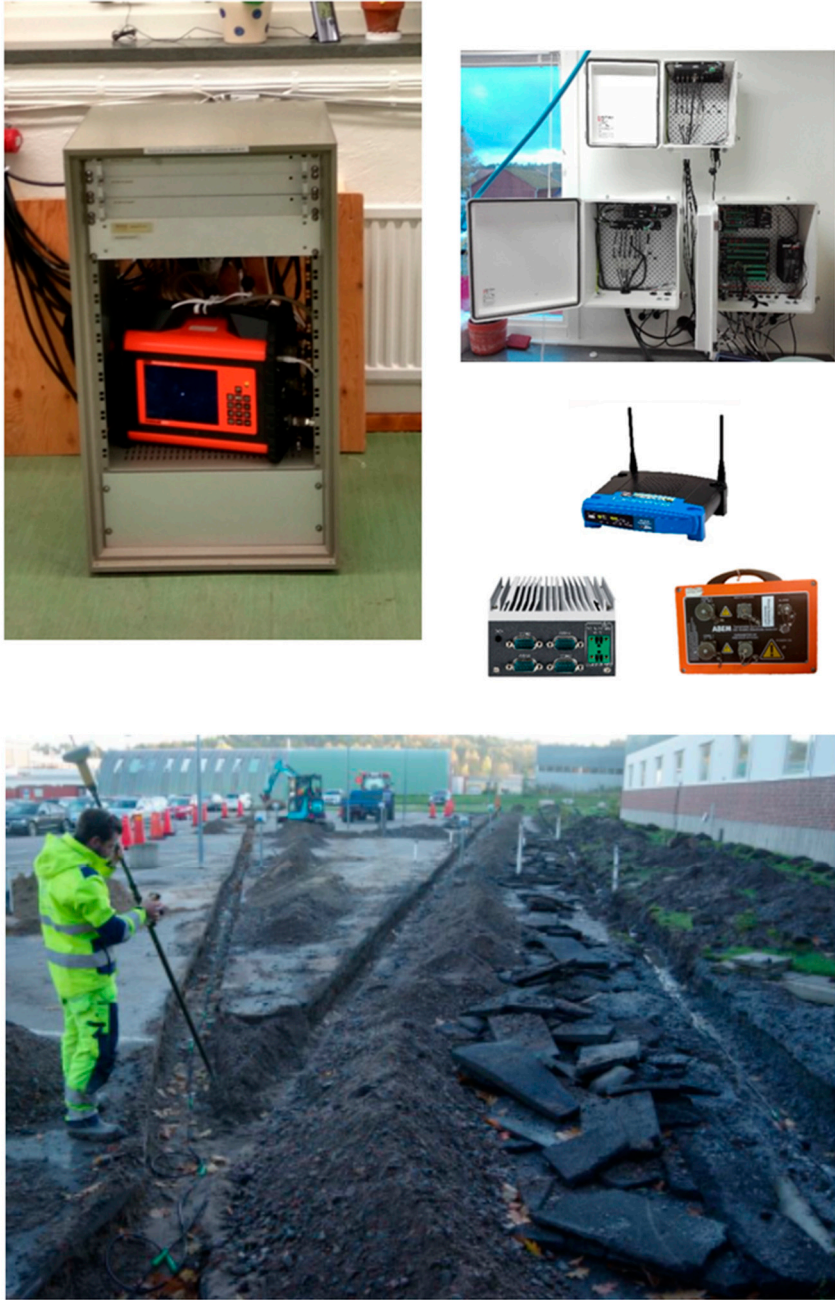
Figure 13. Permanent monitoring system installed in Alingsås. Hardware (top) and geophysical installations (bottom).
