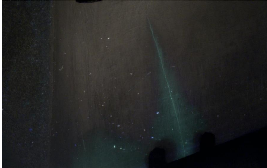
Figure 31: Crack in blade A-19 that spreads from LE to base material of blade outside of the repair
