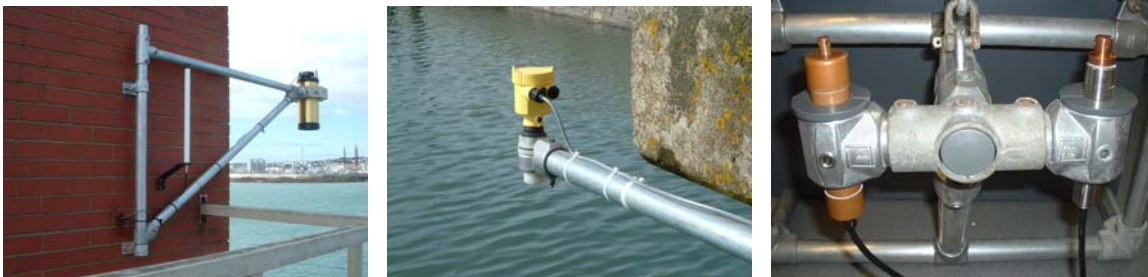
Figure 3. Sensors evaluated at Holyhead were (left) Kalesto radar gauge, (middle) Vega radar gauge and (right) SensorTechnics pressure transducers.
