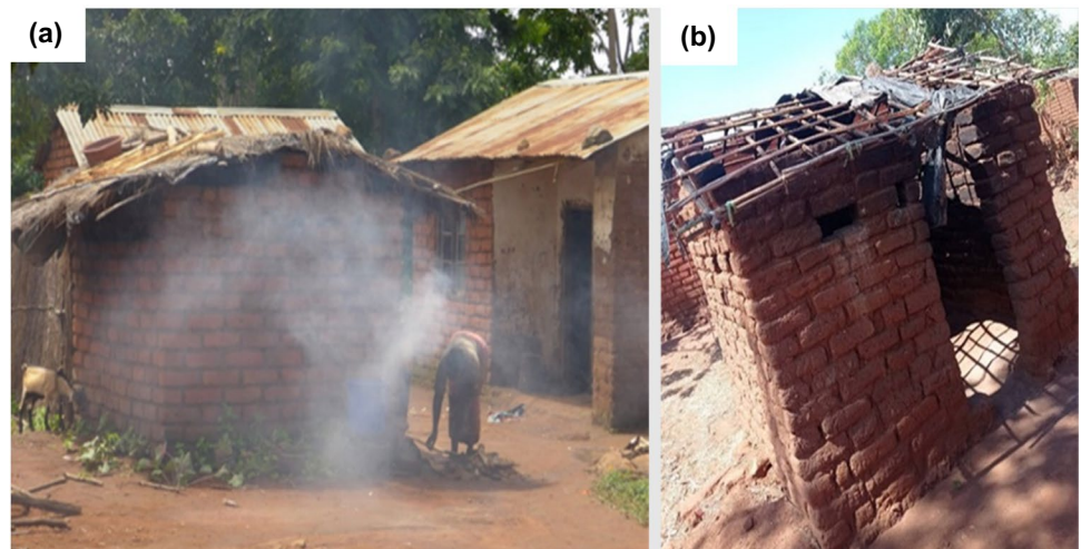
Fig. 5 Sample of kitchen structures in the village: (a) Smoke from a cooking fire started in a separate kitchen. Note the firewood drying on the roof and the smoke vents below the top on the gable wall; (b) The kitchen structure shows an open doorway, roofless and omitted bricks
