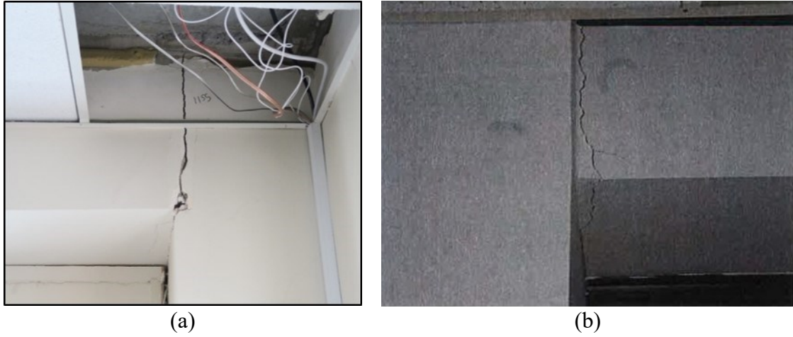
Fig. 1 – Single-crack plastic hinge length after the (a) Kaikoura earthquake; (b) Christchurch earthquake (Photos by Synge A and Smith and Devine (2012))
