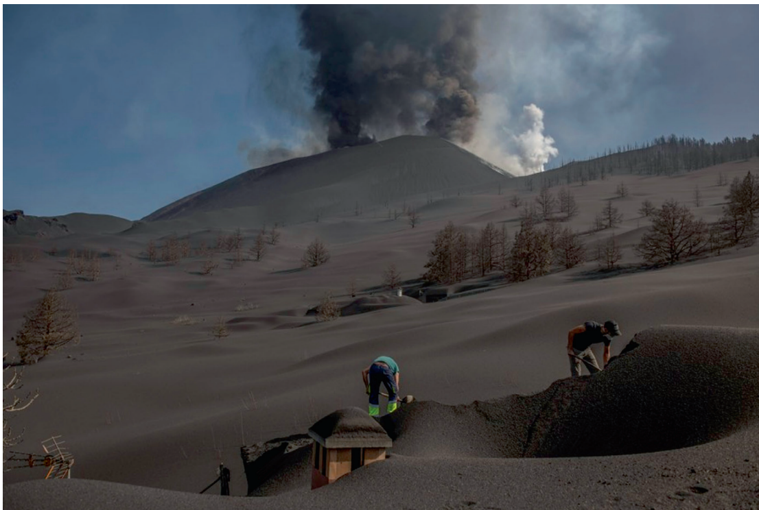
Fig. 1. Workers use shovels to remove volcanic ash that has piled on top of a house in Las Manchas on the Canary Island of La Palma, Spain, on 14 October, 2021. Eruptions are continuing in the background, and the volcano was only declared dormant at the end of December 2021. (Source: Saul Santos/AP.)
