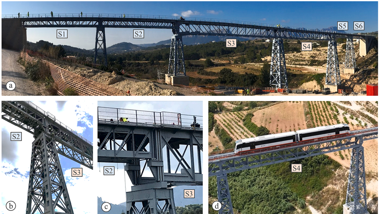
Fig. 1. (a) General view of the bridge; (b) steel pier between spans S2-S3; (c) detail of isostatic span support on a short corbel; (d) train on span S4 during a load test.
