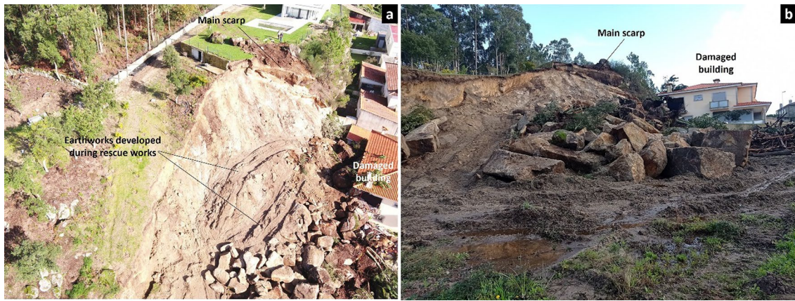
Fig. 1 (a) Aerial and (b) ground general views of the rock planar slide that occurred in Esposende on November 23, 2022
