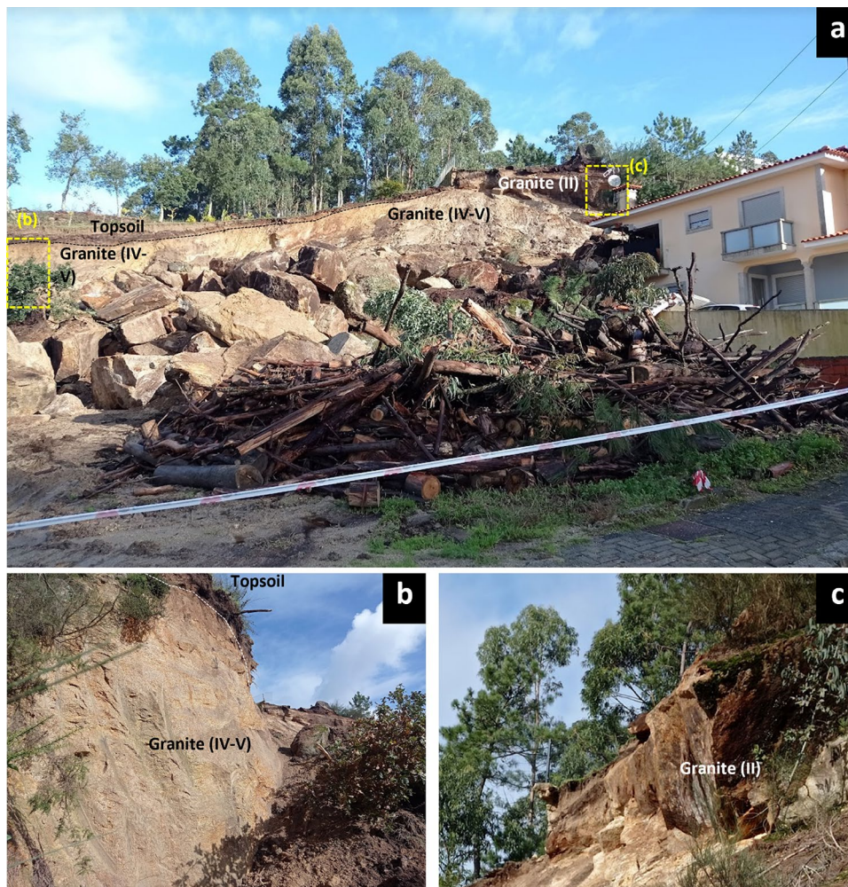
Fig. 3 (a) Geology of the slope. (b), (c) Detail of the different defined lithological units. The weathering degree is expressed in Roman numerals into brackets. Notice tooth marks from the bucket of a mechanical excavator in the slope on (b) evidencing the high weathering of the granite in some parts of the slope
