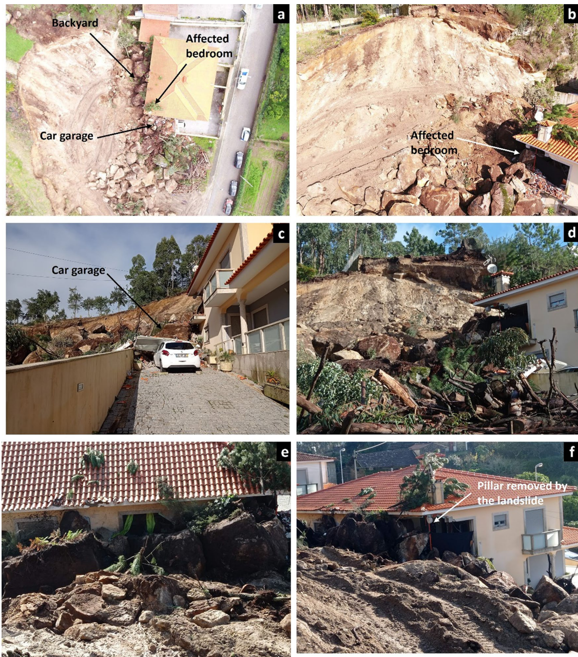
Fig. 4 Picture of the damage caused by the rock planar slide on the building placed on the foot of the slope. (a) Plan view showing the different elements affected. (b) Oblique image of the affected building and the room in which the two deceased people were sleeping. (c) Car garage buried by the landslide. (d) Front image of the rock planar slide and the room impacted by the landslide. (e) Rear façade of the building in which the three bedrooms were placed. (f) View of the part of the building struck by the landslide in which the removed pillar and enclosure of the affected bedroom can be observed
