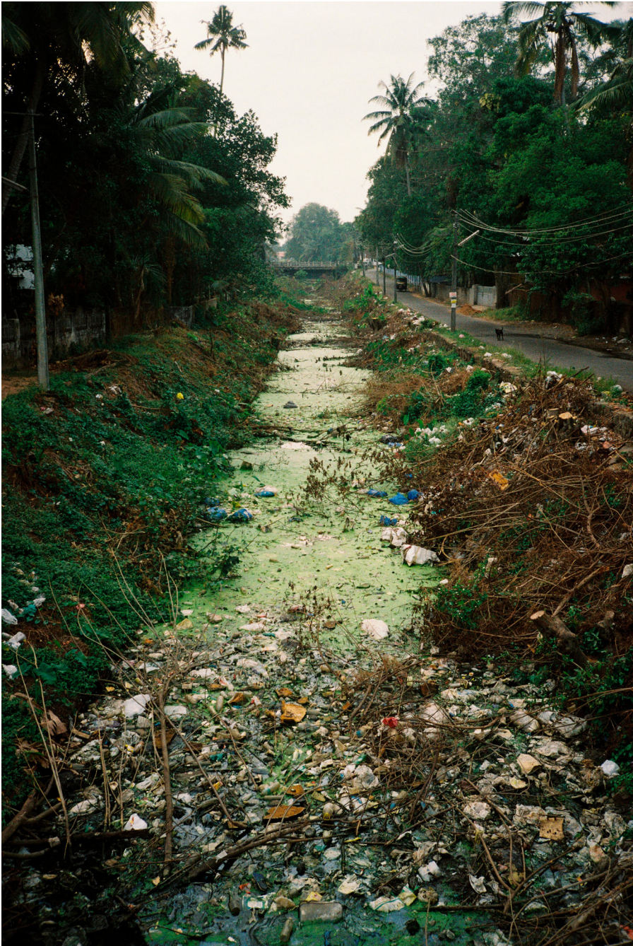
Figure 1 A plastic-clogged canal in suburban Kochi. Photo by Matt Barlow.
