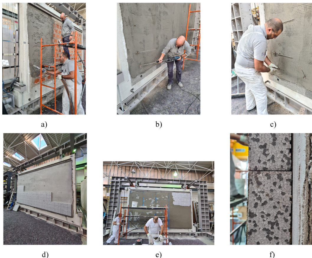
Fig. 5. Retrofitting process of specimen ES_2: a) application of a first layer of mortar; b) connectors application; c) Connectors positioning process; d) application of EPS plates; e) application of nonstructural mesh; and f) profile view of the retrofitting layers.
