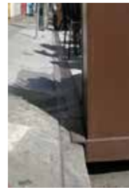
A flush transition at the sidewalk and curb San Francisco, CA, Credit: Nelson\Nygaard
