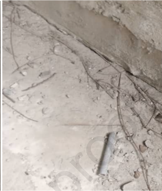
Fig. 13. Crack on joint between wall and floor.
