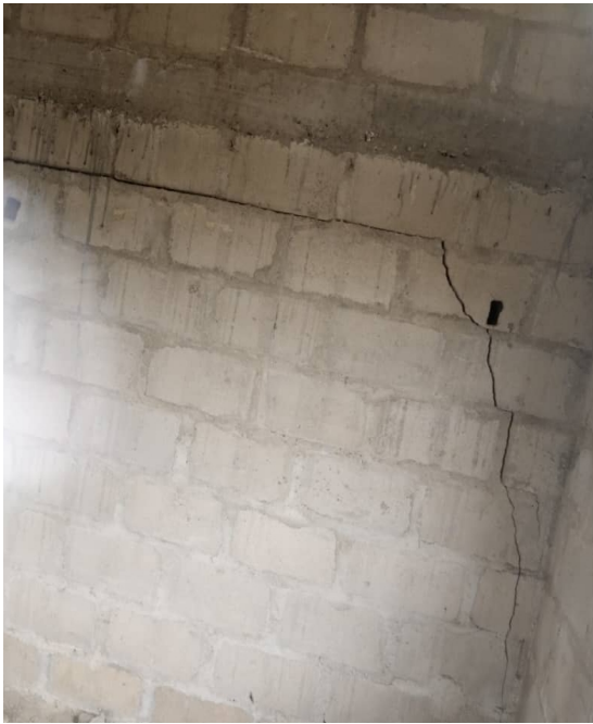
Fig. 12. Cracks noticed on walls
