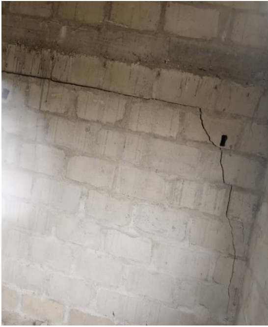
Fig. 12. Cracks noticed on walls
