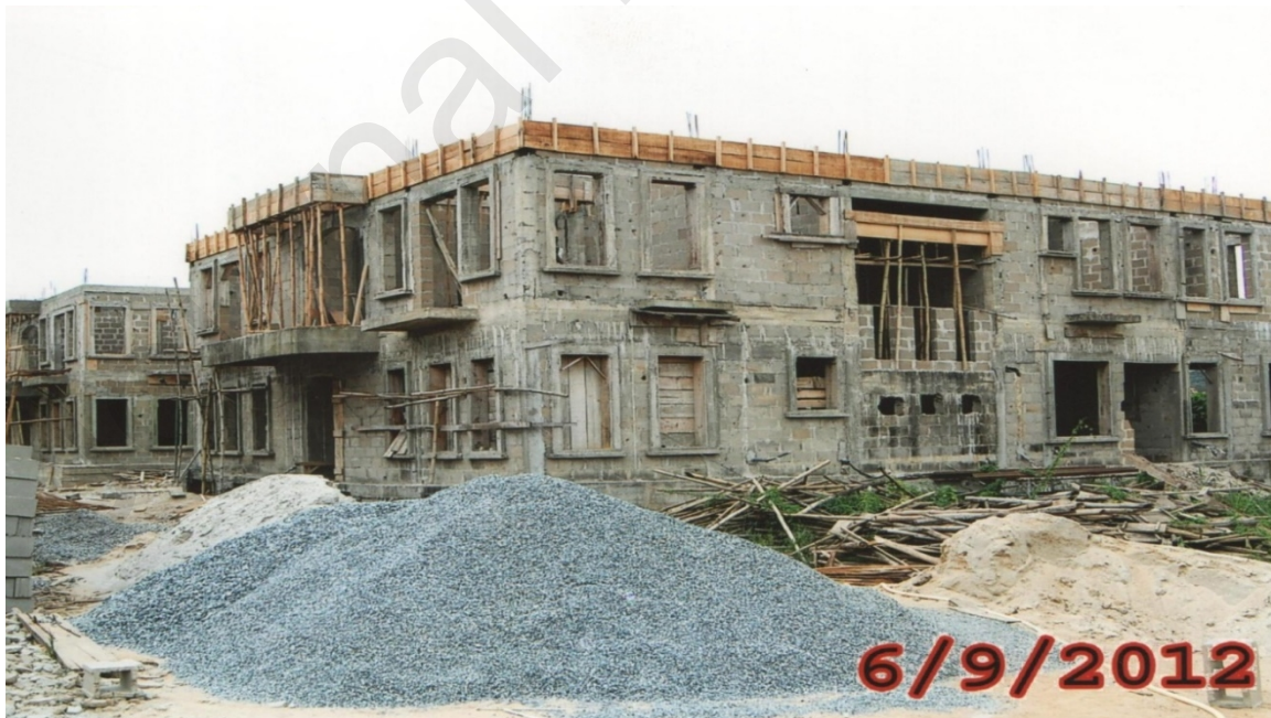
Fig. 11. Distressed building in 2012
