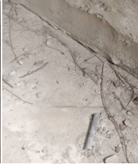
Fig. 13. Crack on joint between wall and floor.
