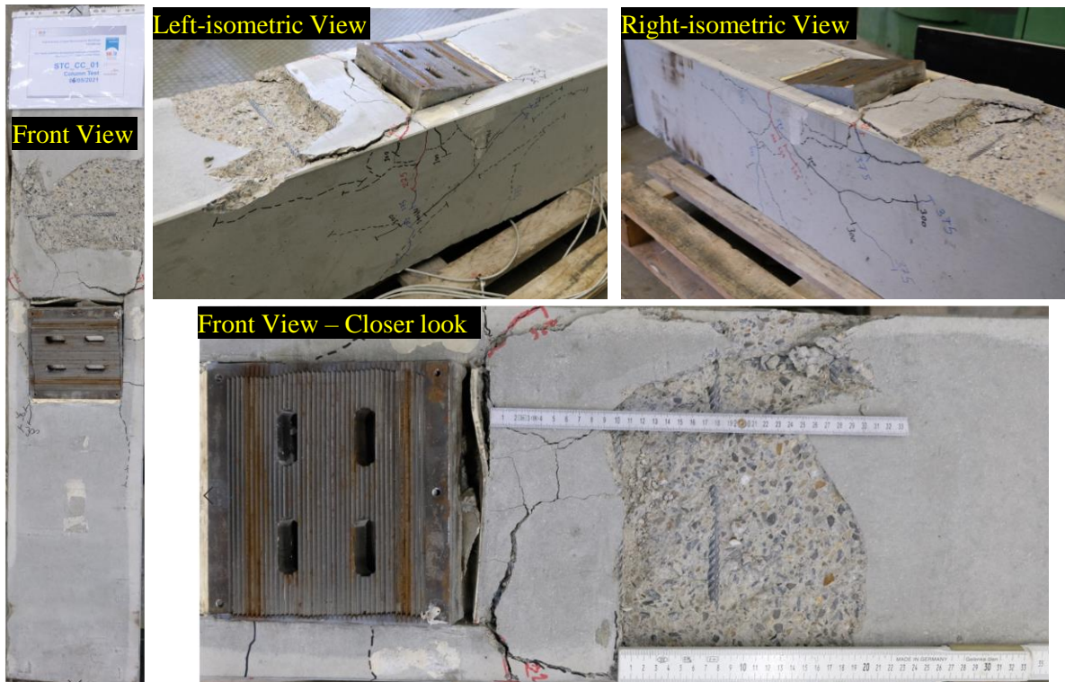
Figure 3.50: Crack patterns after the disassembly of the set-up components / CC-01.
