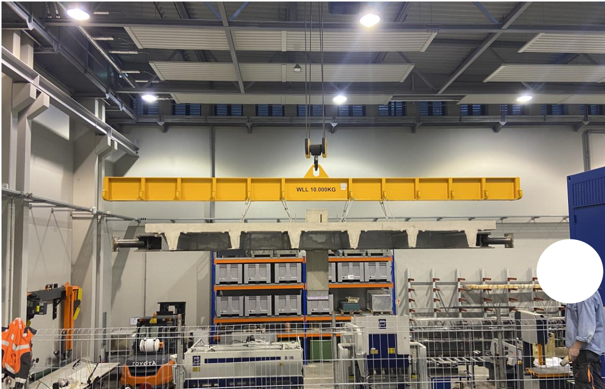
Installation of the Temporary Supports and the Preparation for the Upside-down Turning Operation
