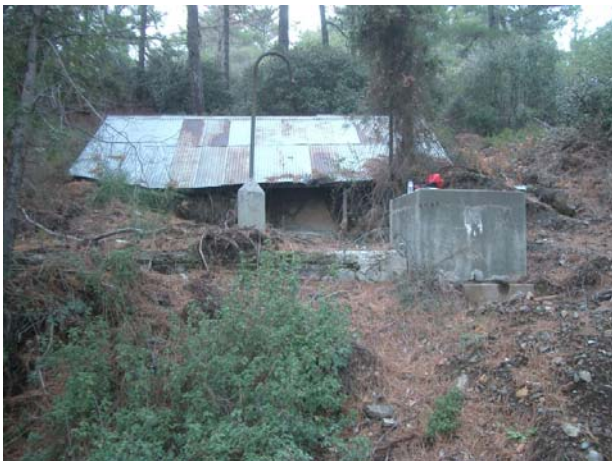
FIGURE 5: THE ORIGINAL SPRING AT SITE C2 (CHRISOVRYSI SPRINGS) IS UNDER THE OLD ROOF AND GROUNDWATER LOOKS TO HAVE FLOWED THROUGH THE SOILS AT THE SITE (NUMEROUS TUFF VEINS CAN BE SEEN THROUGH THE SOIL). FROM ALEXANDER AND MILODOWSKI (2009)
