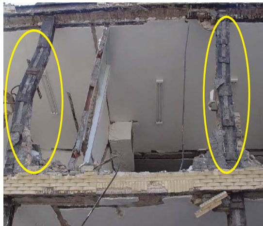
Global buckling of columns
