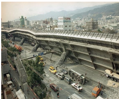
(c) Flexural and Shear failure of an expressway columns 1995 Kobe earthquake (4)
