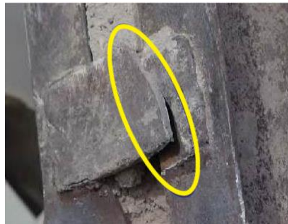
Fracture of battens
