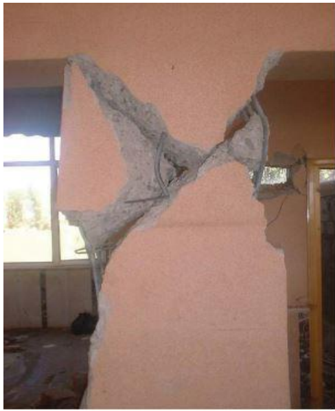
(a) Diagonal tension failure in columns, in an Earthquake in Turkey (2)
