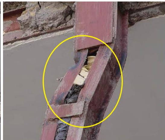
Local buckling of column
