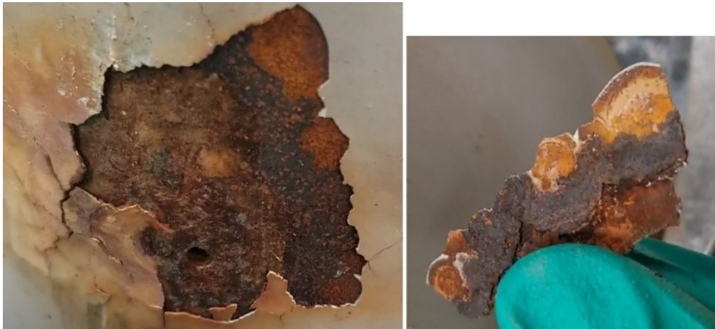
Figure 4.14: Corrosion under coating of 13C. SEM performed on epicenter of break until right edge of coating still attached. See Figure 4.15 to Figure 4.21.
