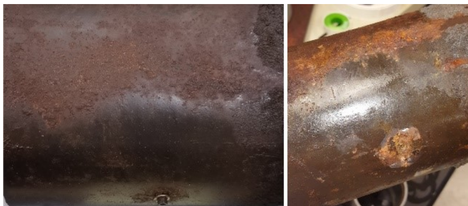
Figure 4.23: Pipe 3B in July (left) and December (right)
