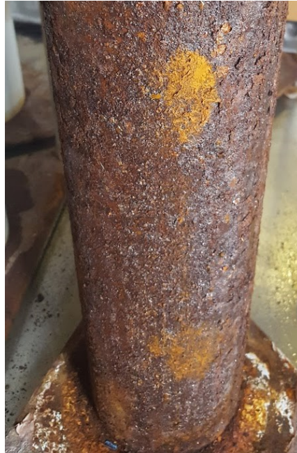
Figure 3.5: IUP pipe 26 June 2017, underwent significant CUI compared to others when inspected. Lightly bound oxide and exfoliation was over the entire surface.
