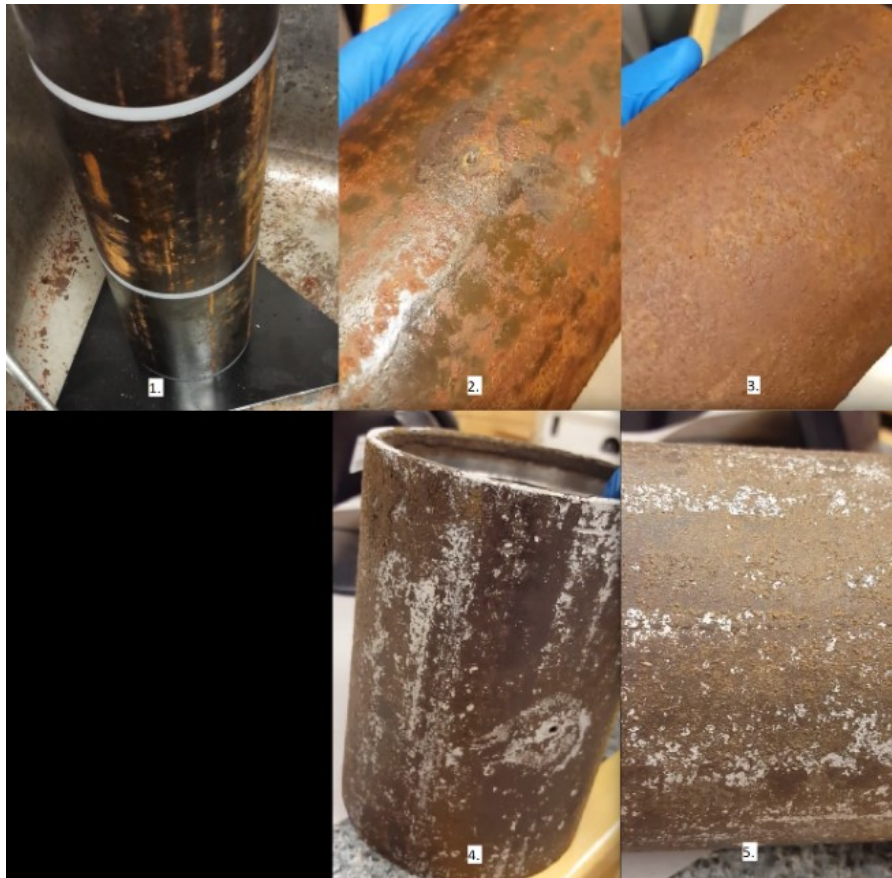
Figure 3.4: 1.) Pipeline 2, in top left initial condition Fall 2015, 2.) to the immediate right top and 3.) to the second right top Pipe 2 during Fall 2016, 4.) bottom center and 5.) bottom right after cleaning Fall 2016.
