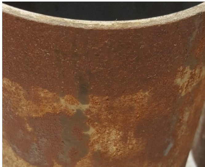
Figure 4.4: Pipe 2B in July showing thin compact oxide layer.
