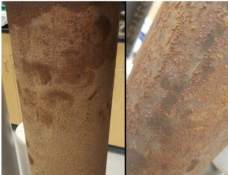
Figure 4.1: Pipe 27 showing compact light layer of surface oxide in patches. Left July, right December.
