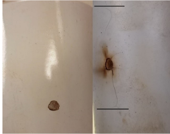
Figure 4.9: Pipe 20, July (left) vs December (right). Coating failure led to corrosion under coating which spread multiple times its initial size under the coating in 6 months.
