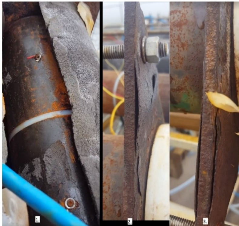
Figure 3.6: 1. One sample opened showing slight corrosion under insulation. 2. & 3. Low carbon steel triangles used for holding pipes together often flaked in large sections as exfoliation.
