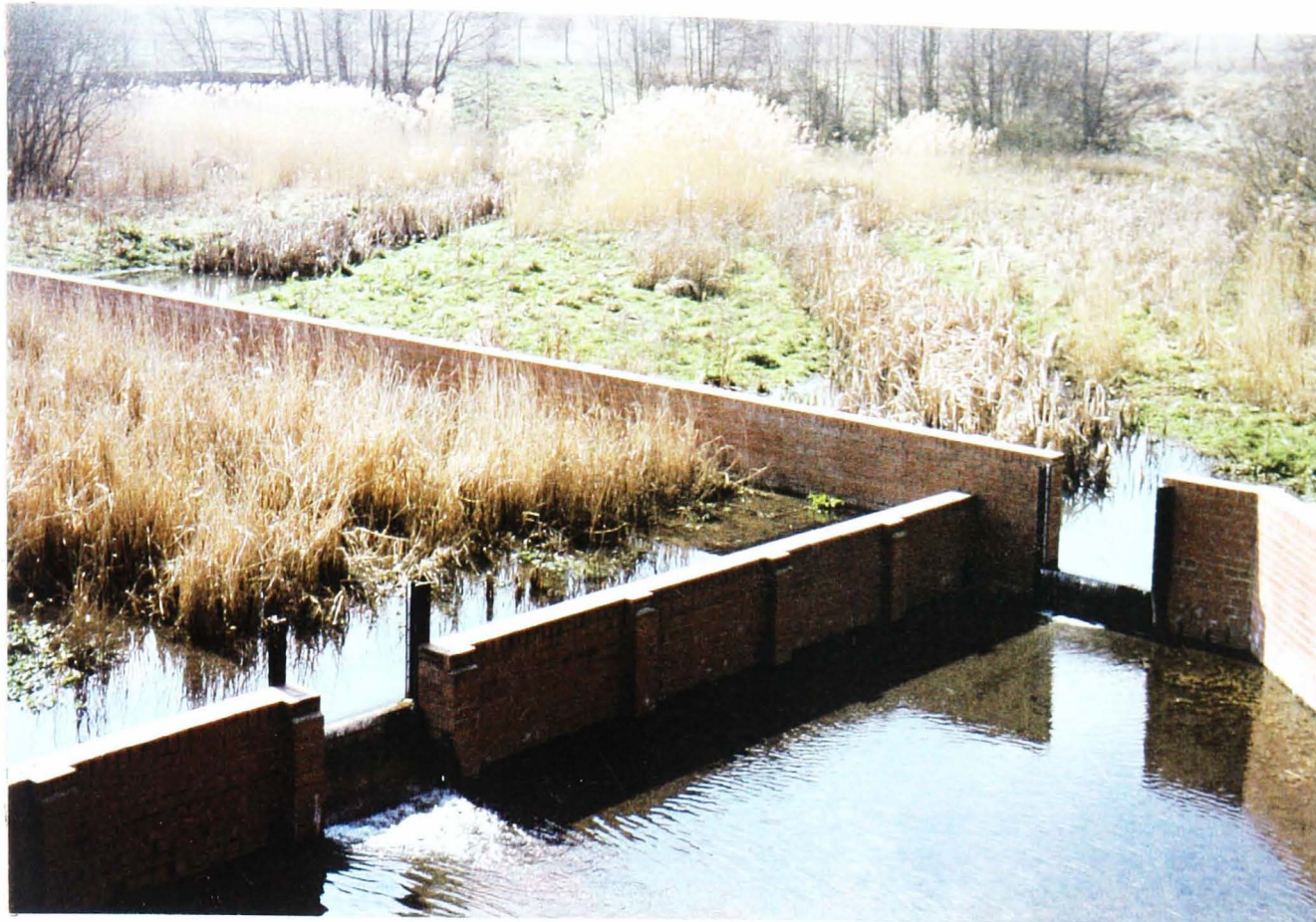
Figure 3. 3 View across final settlement tank looking into the natural wetland component (colonised by Typha latifolia ), Brentwood wetland.
