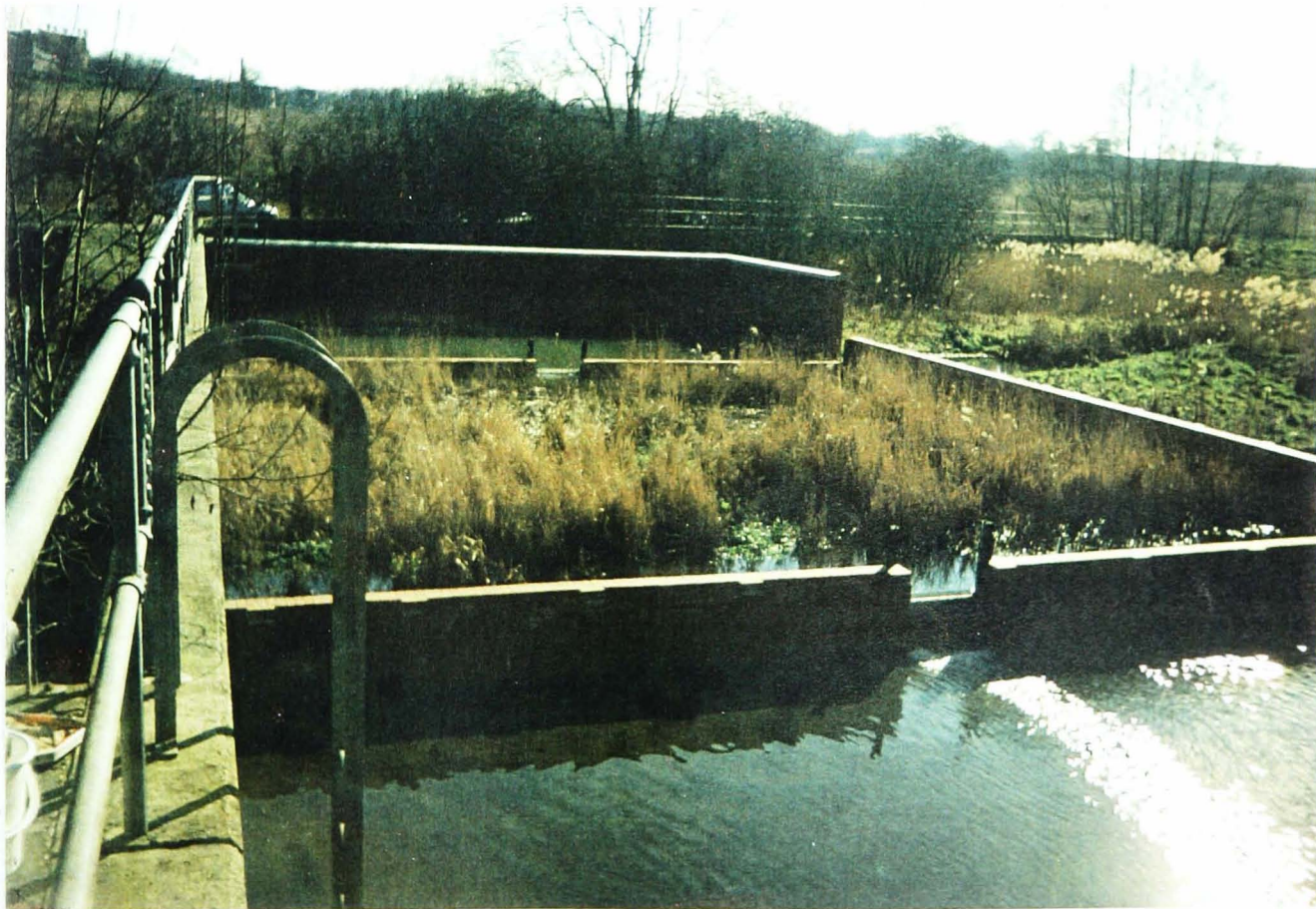
Figure 3. 2 View from the final settlement tank looking back through the constructed wetland component (planted with Phragmites australis ) towards the initial settlement tank, Brentwood wetland.
