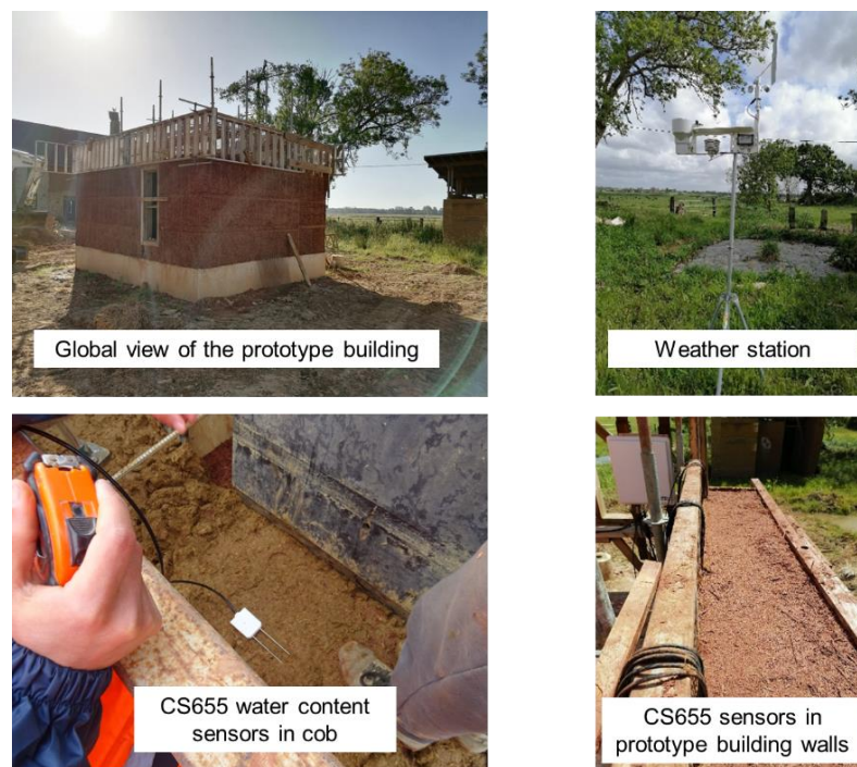
Figure 8. Instrumentation (weather station and volumetric water content sensors) implemented in situ.
