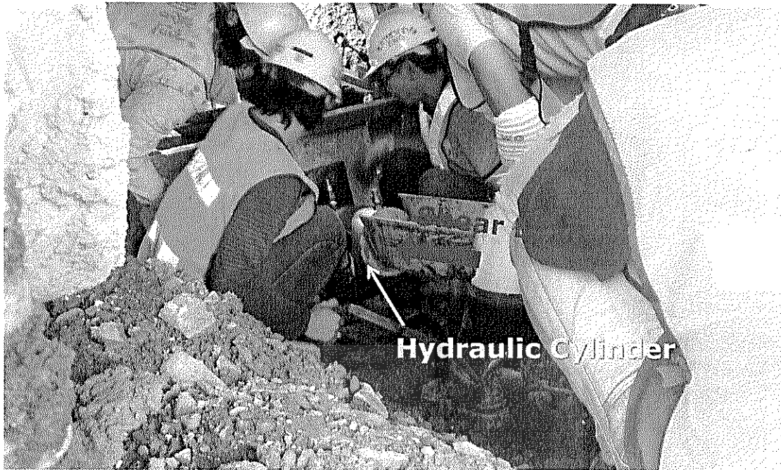
Xayaburi Hydroelectric Power Project, LAOS PDR
