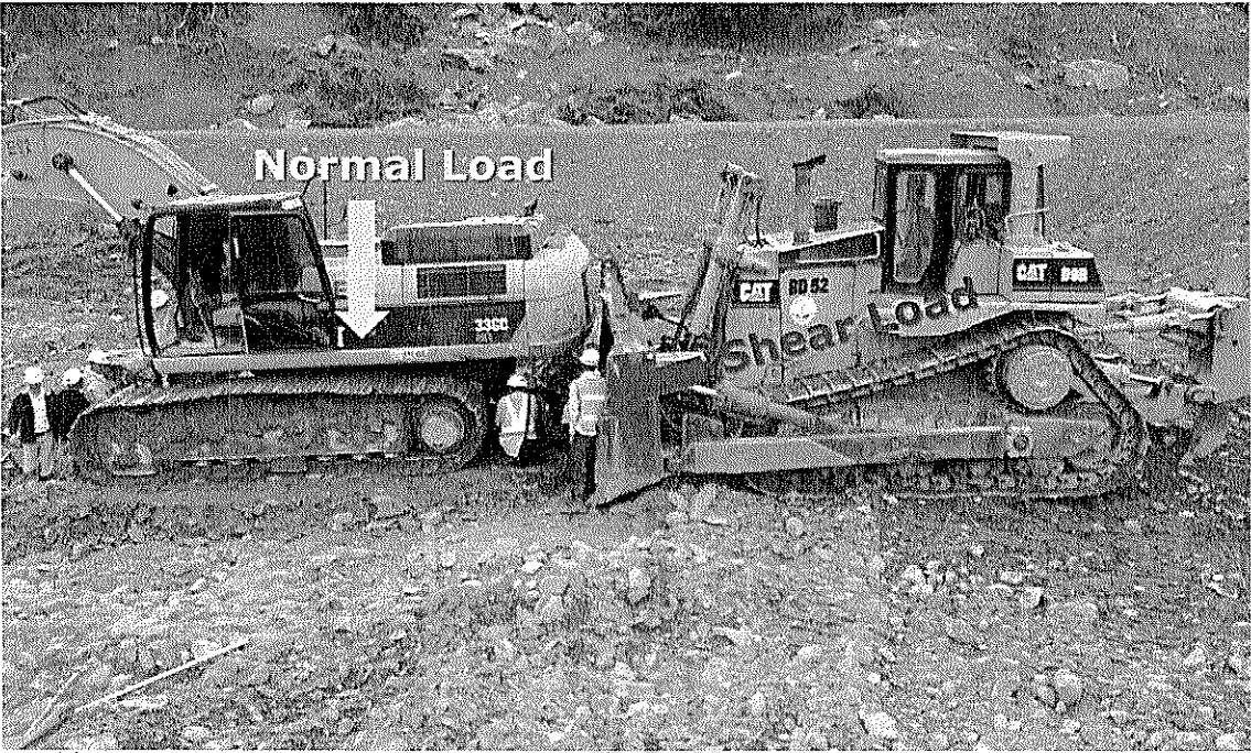
Xayaburi Hydroelectric Power Project, LAOS PDR
