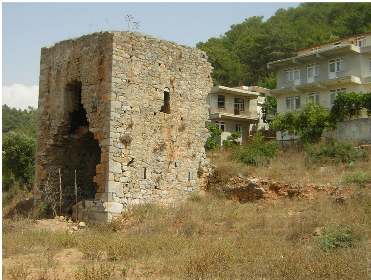
Figure 21: View of Vertical Settings on Side Wall of Tower, Level with Adjoining Terrace, possibly to House Twin Lever Press Arms ( Praela ), Biçkici Kiln Site
