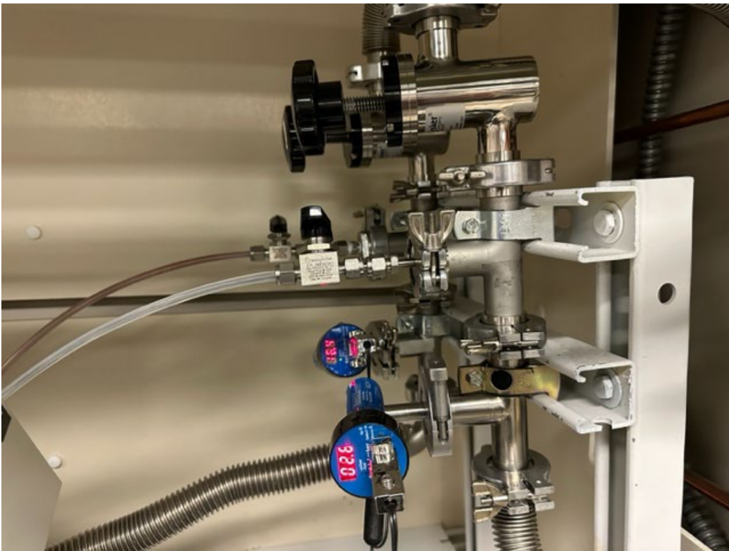
Figure A.2.3: Vacuum and atmospheric valves with pressure gauge.
