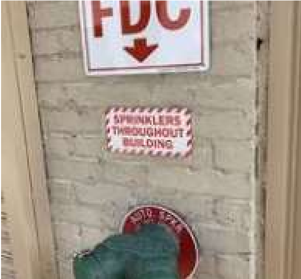
Figure 124: Representative Fire Department Connection for Riser 1.
