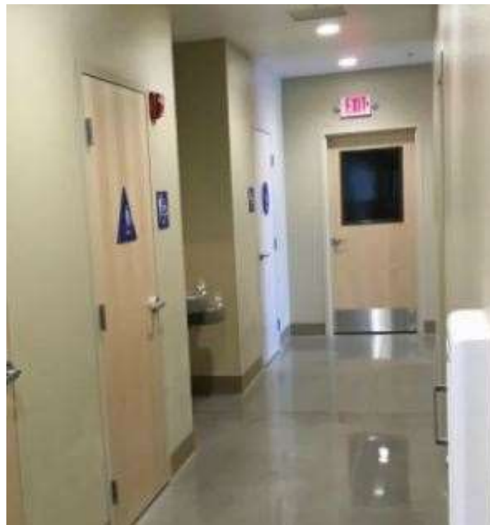
Figure 10: Door #112. This door opens against the flow of egress.
