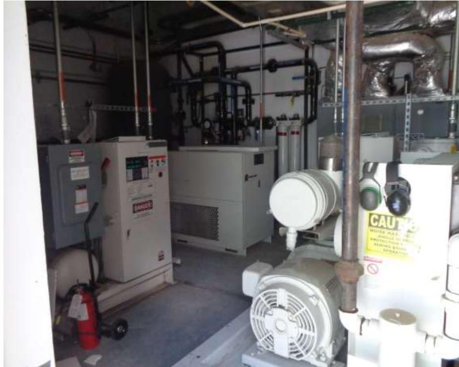
Figure 49: Compressor room on the south side of the ACME Building behind Door S-61U.
