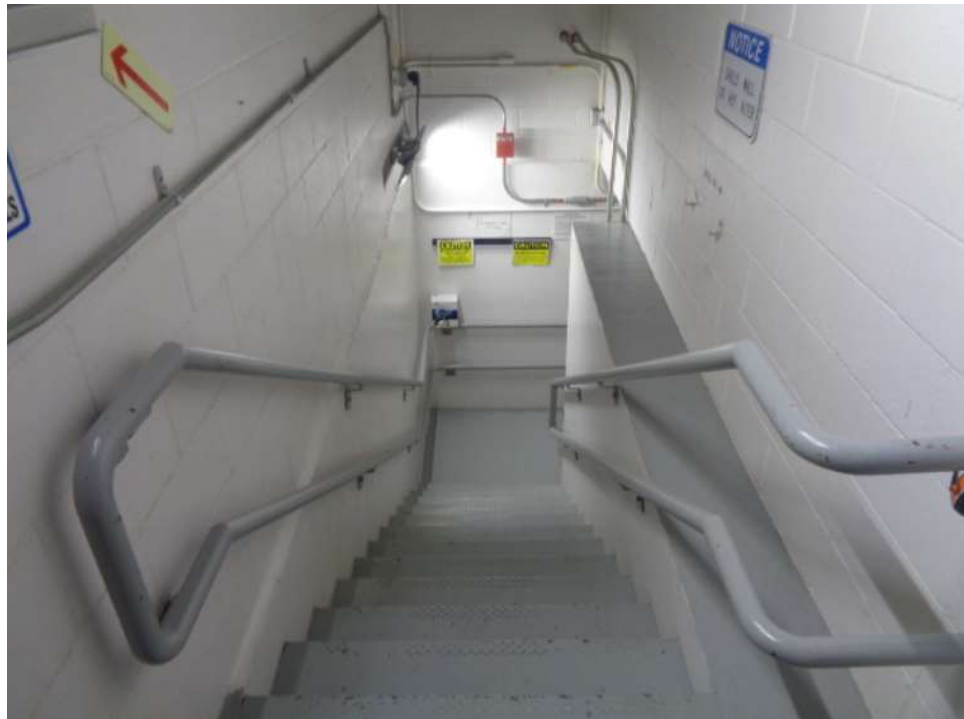
Figure 60: This is the stairway that leads to the CDP elevator equipment pit.
