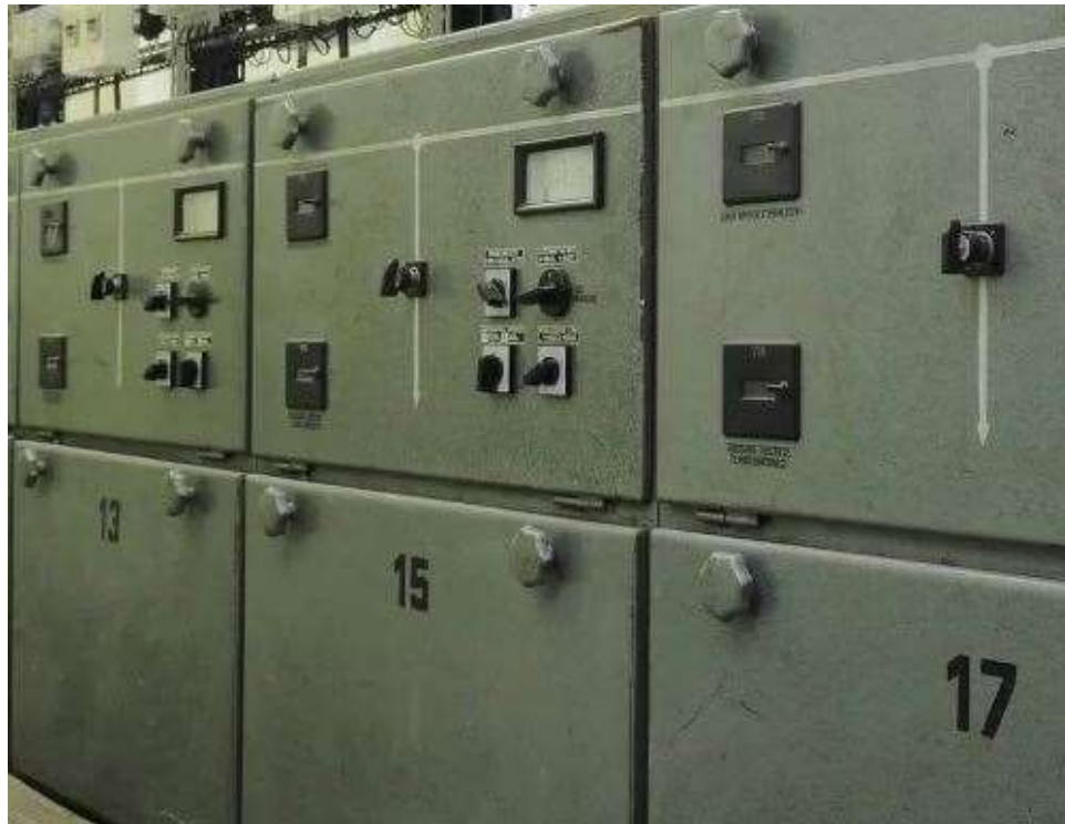
Figure 56: Electrical gear at the west end of the water pool area.
