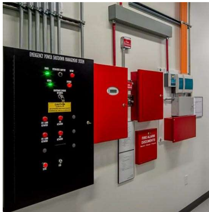
Figure 36: Fire alarm signaling panels near door 112A.
