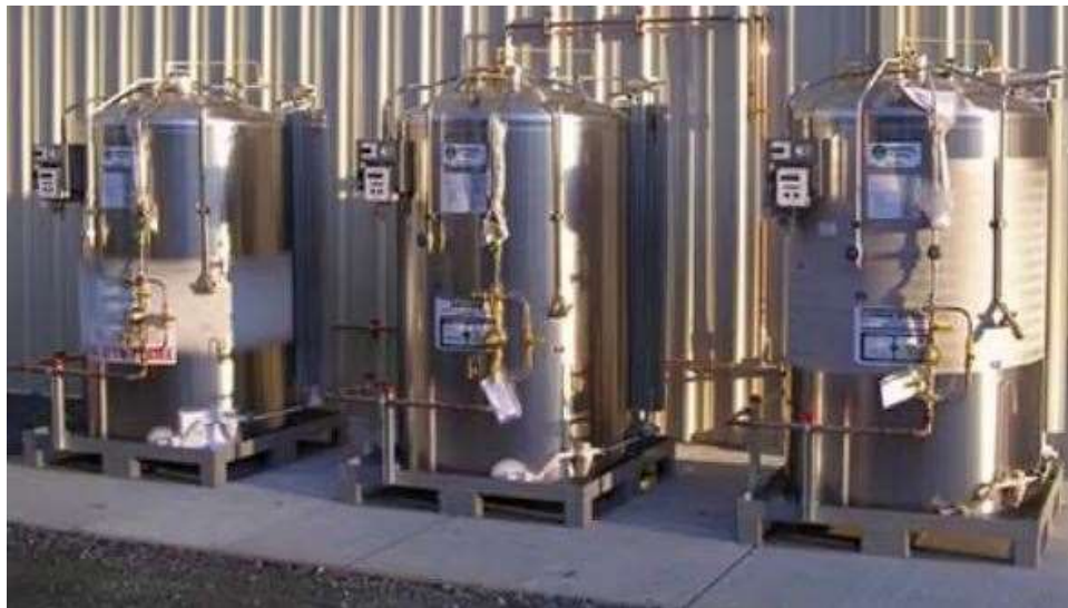
Figure 4: TSA on the north side of the ACME Building that stores compressed nitrogen gas.
