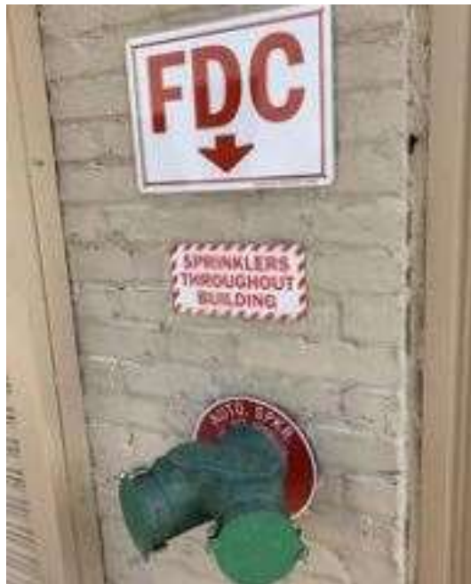
Figure 126: Representative FDC for Riser 3 on the north side of the ACME Building.
