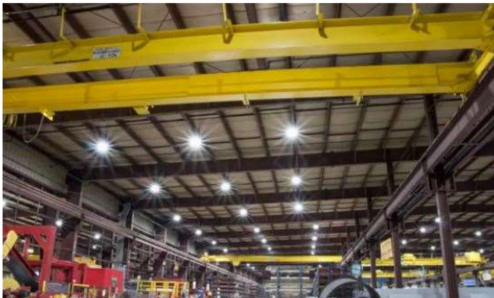
Figure 54: 2 nd floor fan room above the HCOG.
