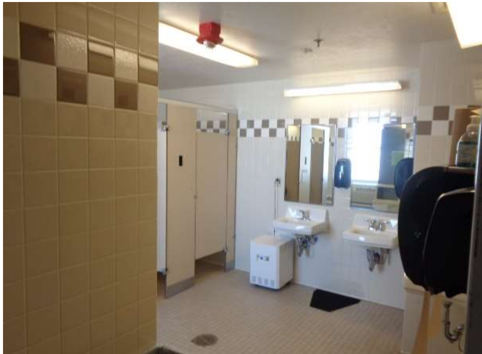
Figure 42: 2 nd floor central men's room on the north side of the ACME Building.
