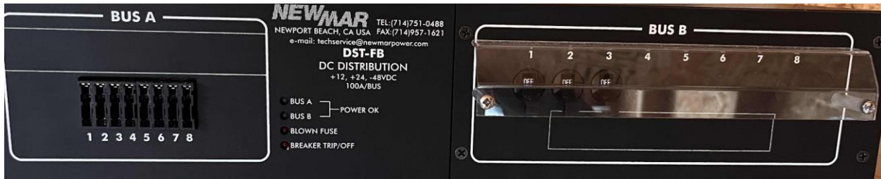
Figure 5.10 Front of NEWMAR DC Distribution.
