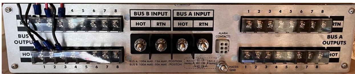
Figure 5.9 Back of NEWMAR DC Distribution.
