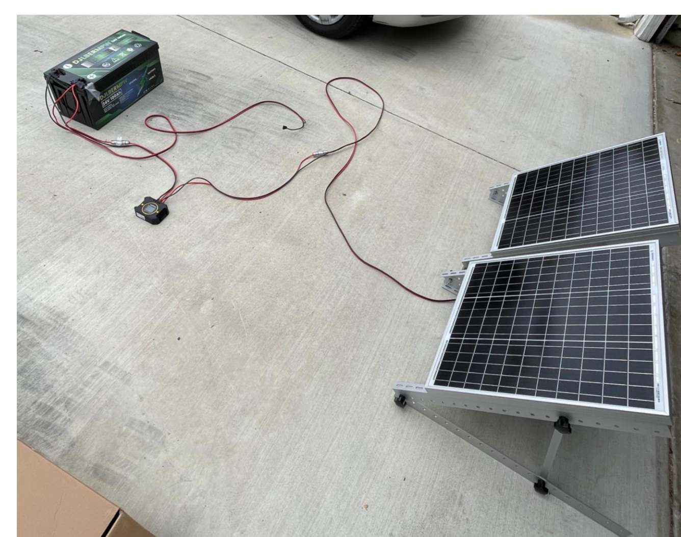
Power Generation & Storage
