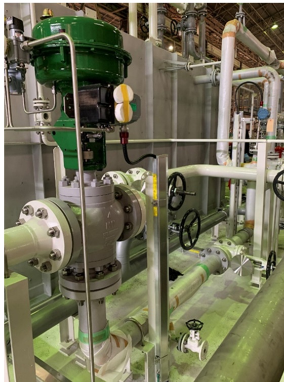
Figure 9: Oil Temperature Control Valve (Image source: Yoshimine, Japan)
