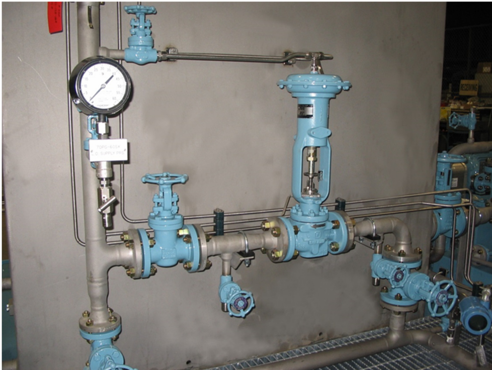
Figure 17: Lube Oil Pressure-reducing Control Valve (Image courtesy of G.J. Oliver, Inc.)
