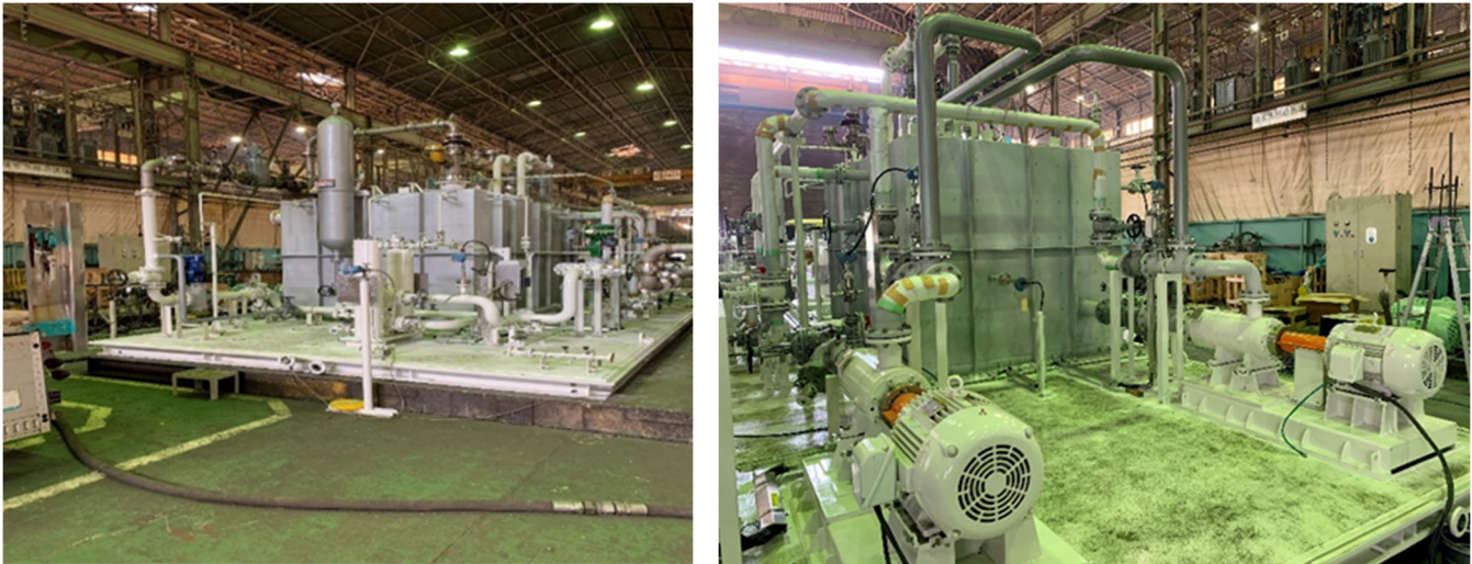
Figure 1: Lube Oil System for a Centrifugal Compressor String (Image source: Yoshimine, Japan)
