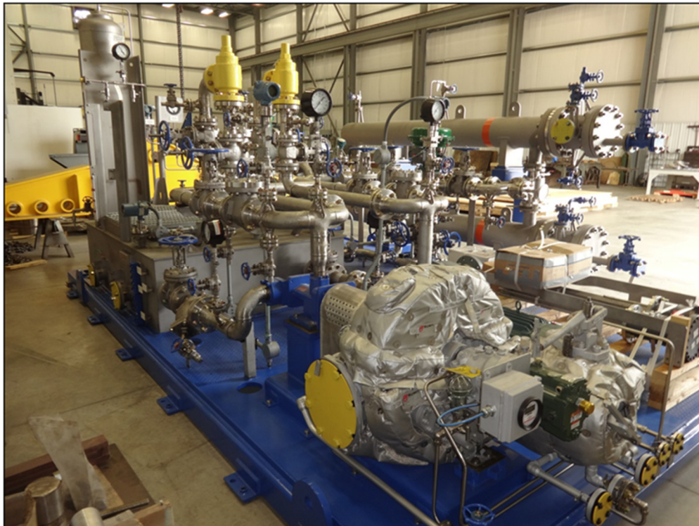
Figure 27: Steam Turbine Driven Main Pump Lube/Control Oil Console (Image courtesy of G.J. Oliver, Inc.)
