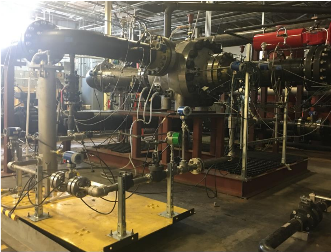
Figure 32: Turbocharger FAT setup with lubrication skid in the foreground
