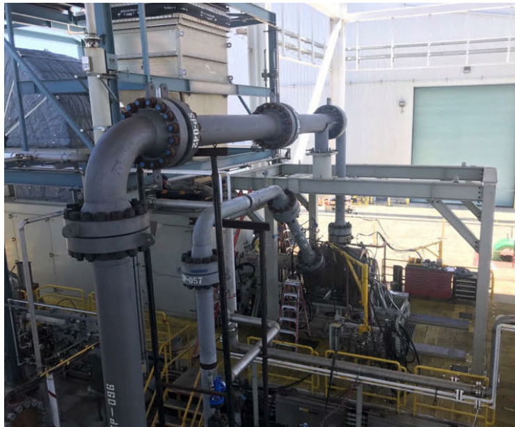
Figure 7a. Closed-loop arrangement of the high pressure compressor
