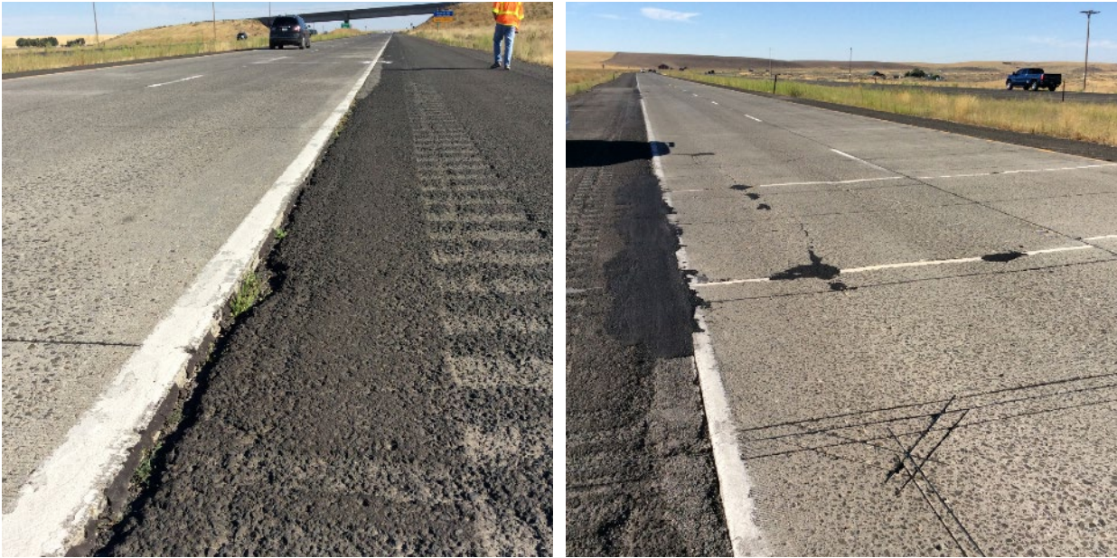
Figure 34. Section 530205, 550 psi, 8" PCC, 6" LCB. August 2017. No tining visible, three transverse cracks with spalling. Some asphalt patching of spalled cracks.
