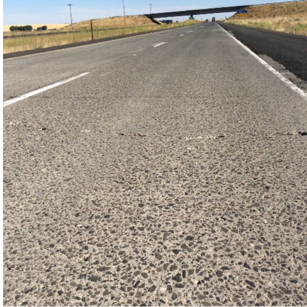
Figure 32. Section 530205, 550 psi, 8" PCC, 6" LCB. August 2017. No tining visible, three transverse cracks with spalling.
