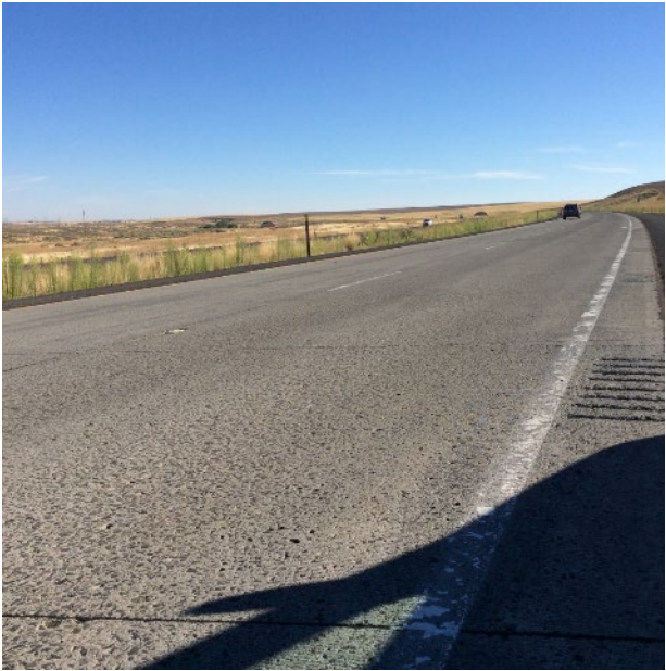
Figure 23. Section 530259, 650 psi, 10” PCC, 3” ATB. August 2017. Some tining visible, no cracks or spalls.
