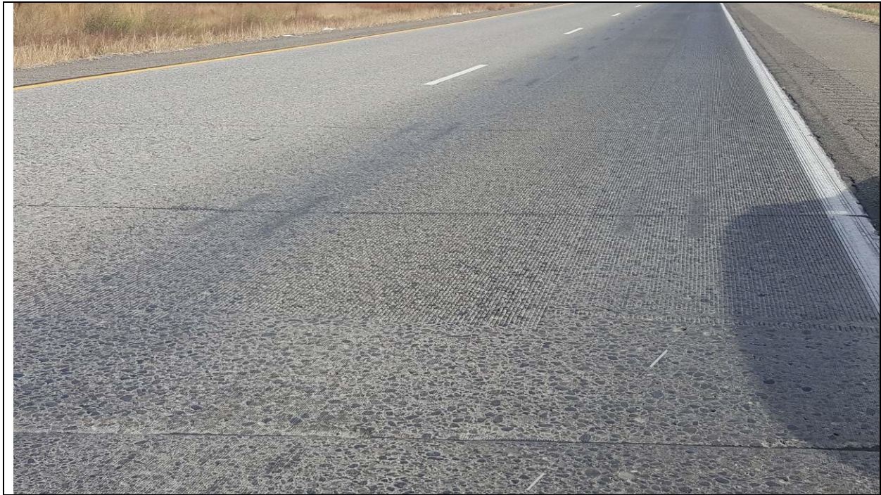
Figure 4. Transition between CDG foreground and NGCS background. Note slight spalling at the transverse joints. October 2017.
