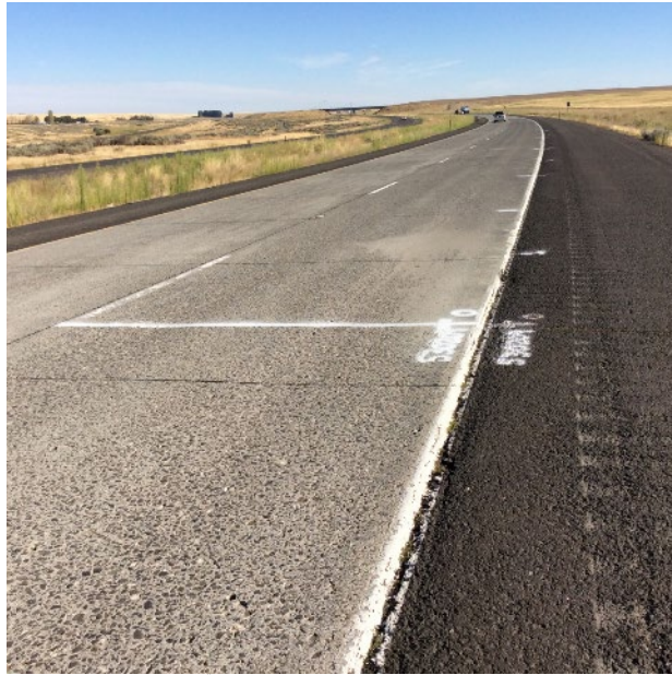
Figure 28. Section 530209, 550 psi, 8” PCC, 4” PATB, 4” DGAB. August 2017. No tining visible, no cracks or spalls.
