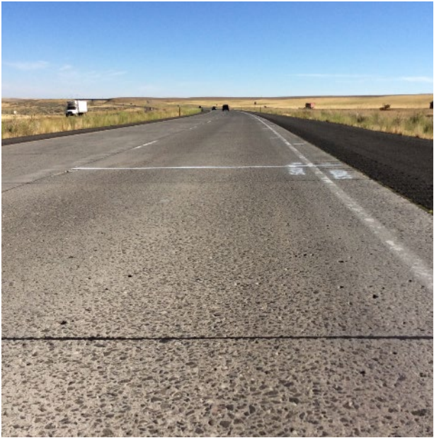
Figure 27. Section 530211, 550 psi, 11” PCC, 4” PATB, 4” DGAB. August 2017. No tining visible, no cracks or spalls.
