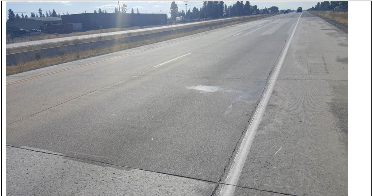
Figure 14. The full lane one inch inlay section of polyester concrete on I-90. (Sept. 2017)
