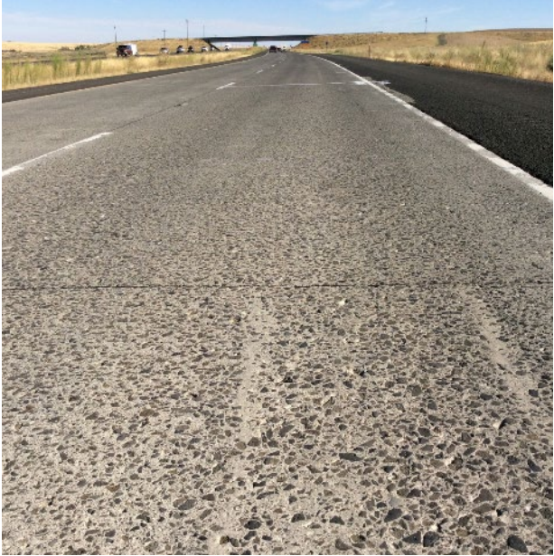
Figure 31. Section 530201, 550 psi, 8" PCC, 6" DGAB. August 2017. No tining visible, two transverse cracks with spalling.
