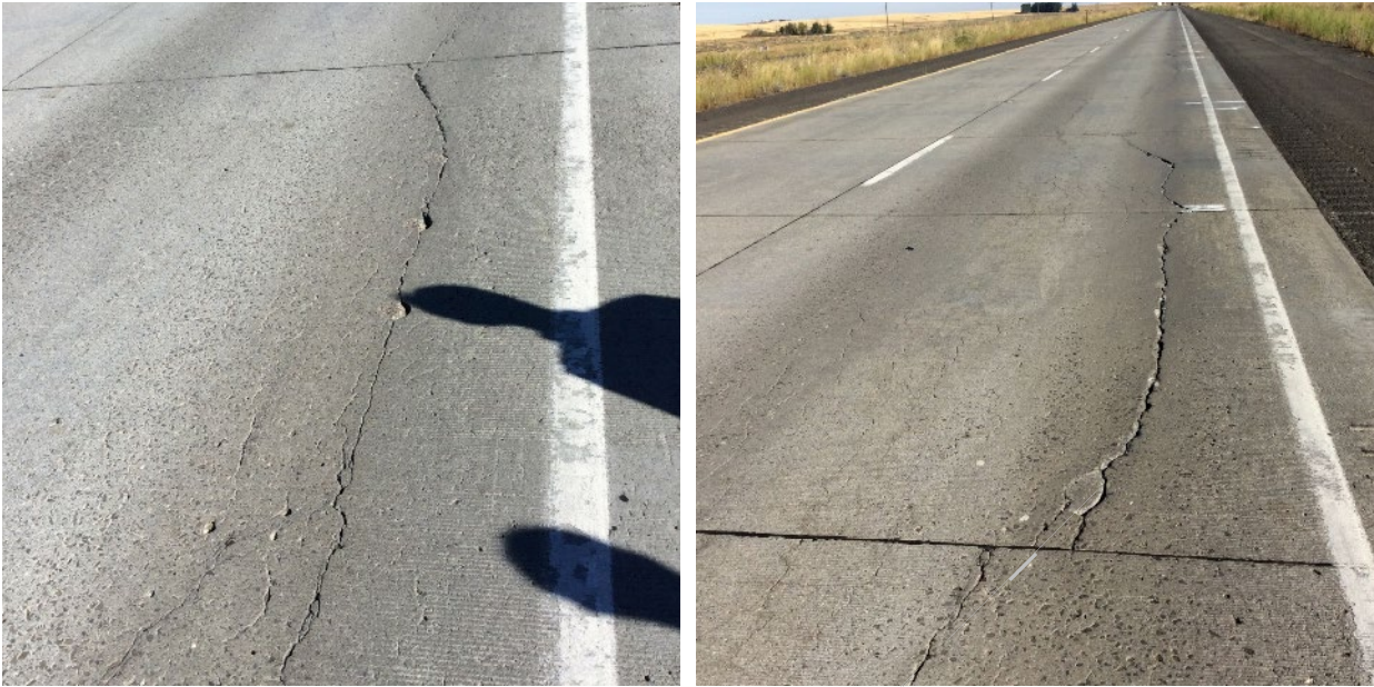
Figure 38. Section 530206, 900 psi, 8" PCC, 6" LCB. August 2017. See Figure 33 for summary of condition statement.
