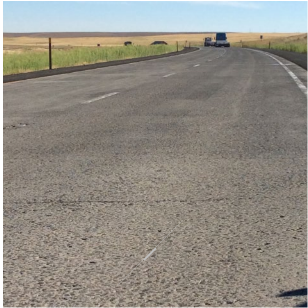
Figure 24. Section 530203, 550 psi, 11” PCC, 6” DGAB. August 2017. Some tining visible, one transverse crack, no spalls.
