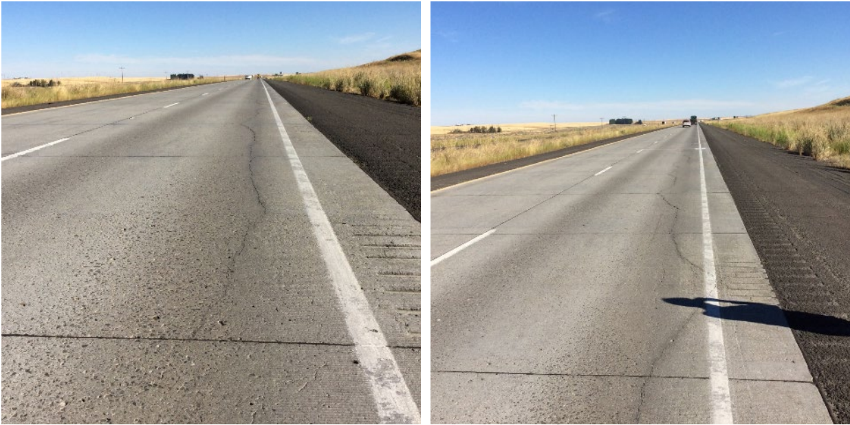
Figure 36. Section 530206, 900 psi, 8" PCC, 6" LCB. August 2017. Some tining visible, longitudinal cracks in both wheel paths that are spalling, appearance of stress induced multi-cracks similar to cracking on bridge decks.
