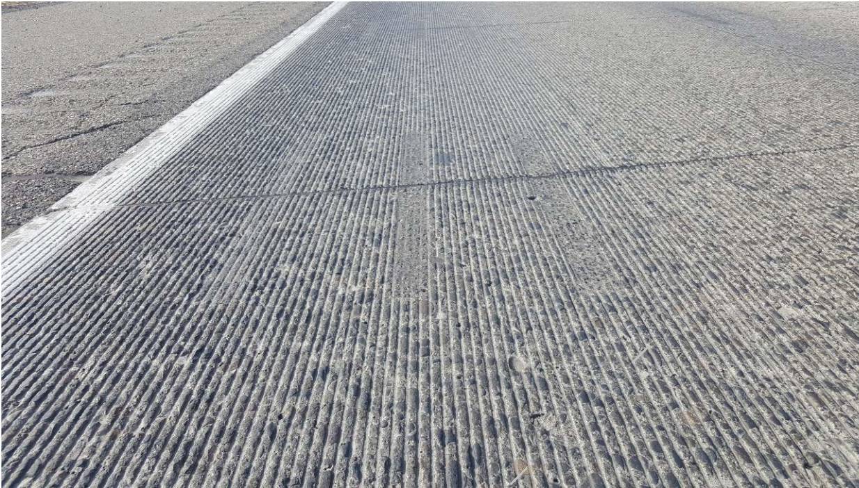
Figure 6. Note erosion of the edges of the land areas on the NGCS and the greater wear on the dowel bar retrofit fill material. October 2017.
