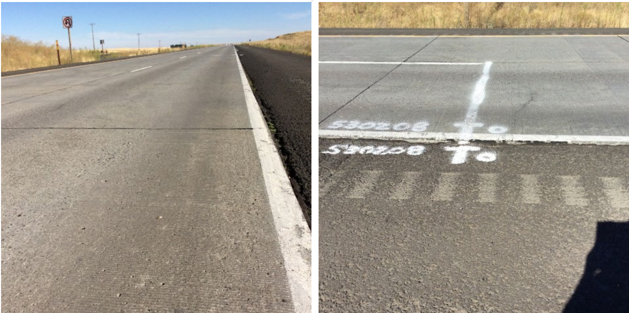
Figure 35. Section 530208, 900 psi, 11" PCC, 6" LCB. August 2017. Some tining visible, transverse cracks and longitudinal cracks in right wheel path.
