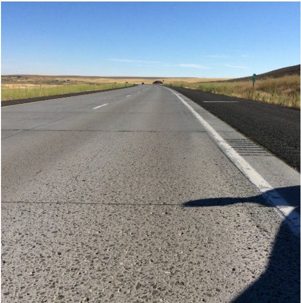
Figure 25. Section 530202, 900 psi, 8” PCC, 6” DGAB. August 2017. Some tining visible, three transverse cracks.
