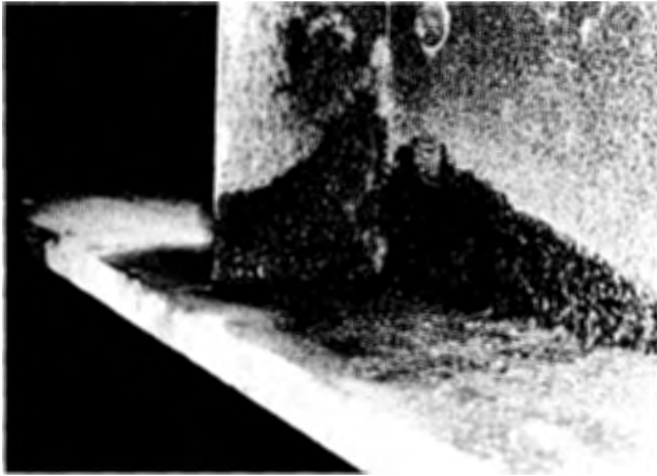
Figure 25. Corroded flange, web, and stiffener welded connection.
