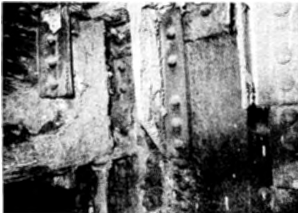
Figure 28. Dirt adhering to stringer and floor beam webs, stringer flanges and end connection angles.
