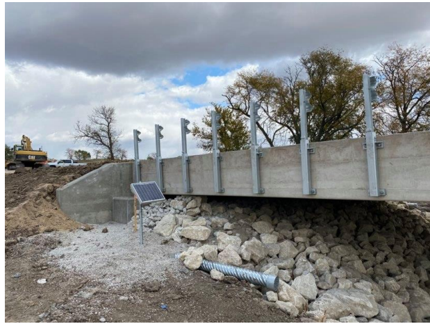
(b) Solar panel
