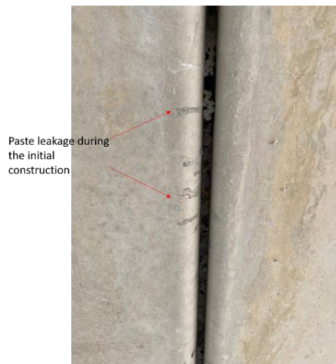
Figure 37. Paste leakage during initial construction
