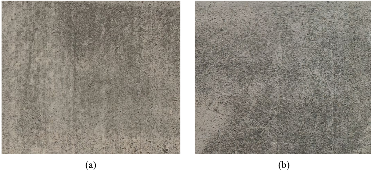
Figure 111. Low- vs Medium-Severity Scaling Detected via sUAS Inspections
