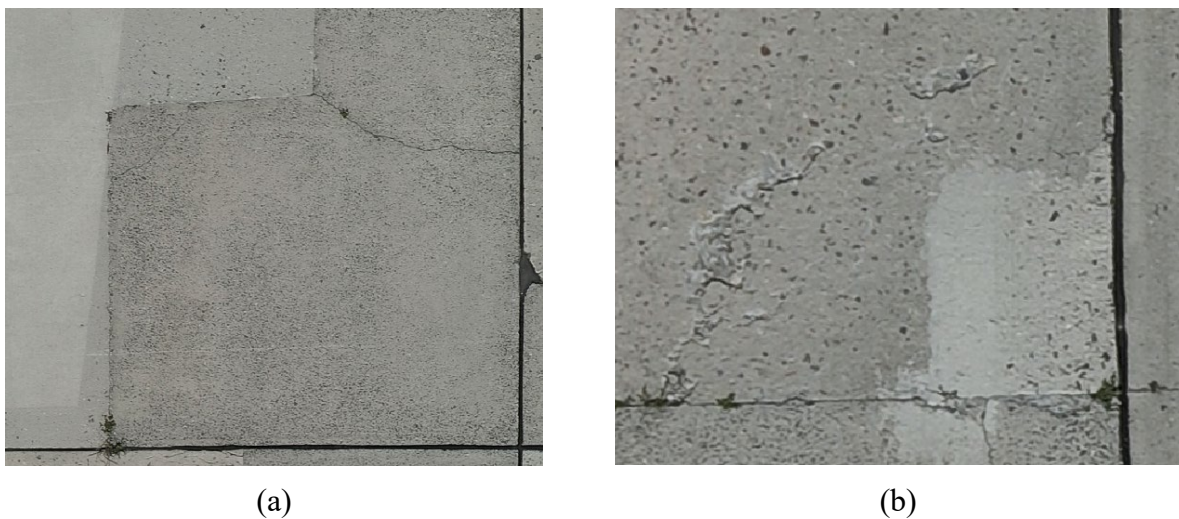
Figure 104. Low- (a) vs Medium-Severity (b) Corner Break Detected via sUAS Inspections
