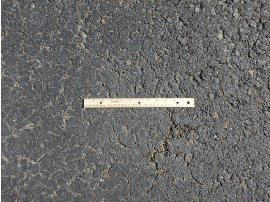
Figure 58. Asphalt Apron Pavement Deterioration at WWD
