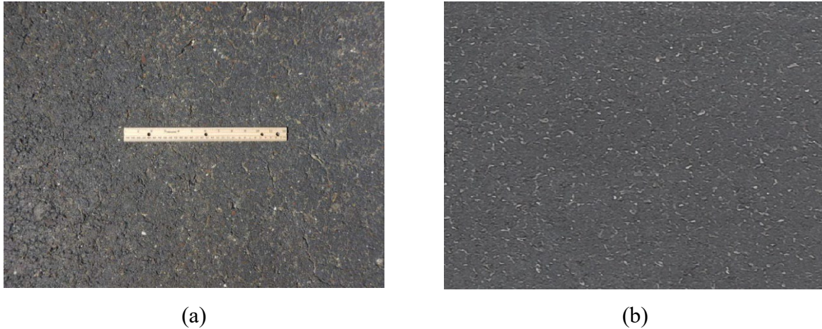
Figure 100. Low-Severity Raveling Detected via FOG (a) and sUAS (b) Inspections
