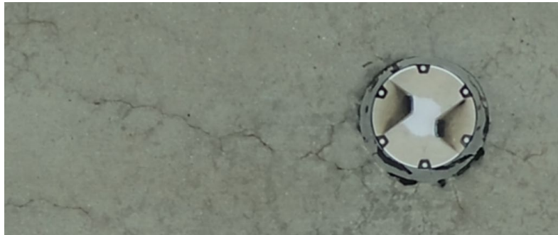
Figure 66. Distress Example on Runway 10/28 at SAV
