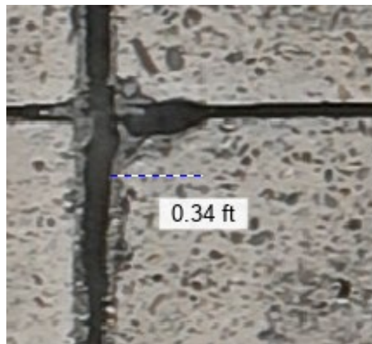
Figure 114. Low-Severity Corner Spall Detected via sUAS Inspections
