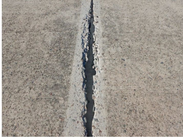
Figure 43. Joint Spall at WWD
