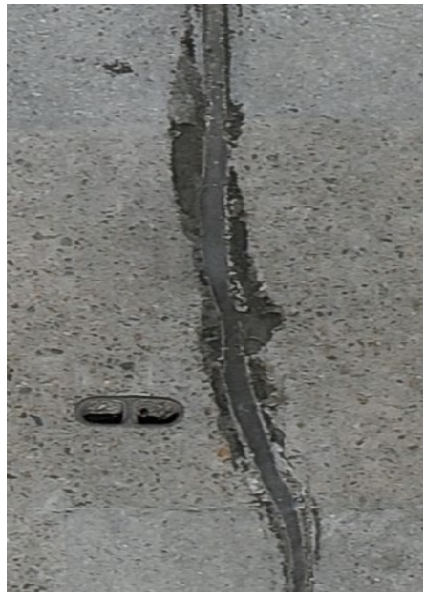
Figure 106. Medium-Severity Linear Crack Detected via sUAS Inspections
