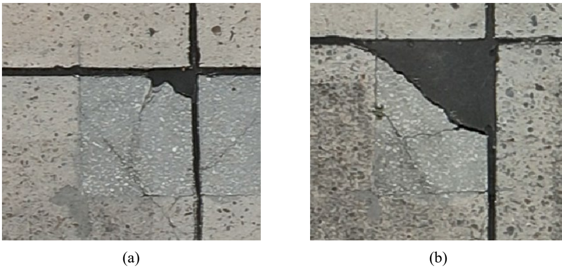
Figure 108. Medium- (a) vs High-Severity (b) Small Patch Detected via sUAS Inspections
