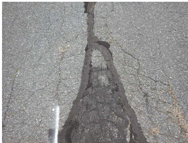
Figure 17. Alligator Cracking Observed on Test Area 2B at WWD
