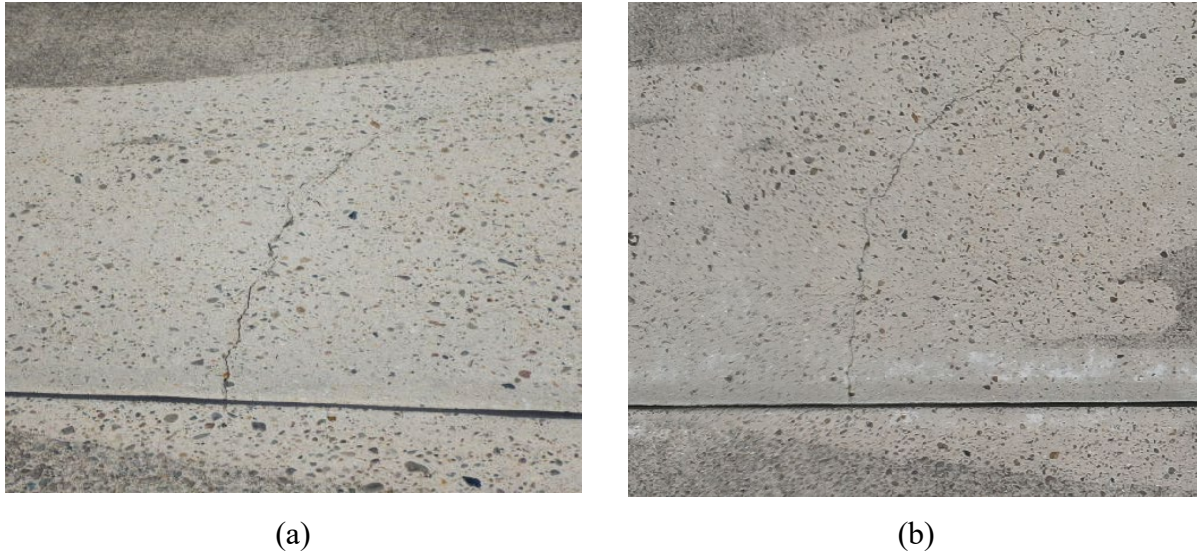
Figure 105. Low-Severity Linear Crack Detected via FOG (a) and sUAS (b) Inspections
