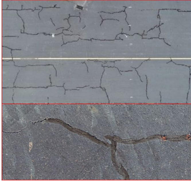
Figure 44. Network of L&T Cracking at WWD
