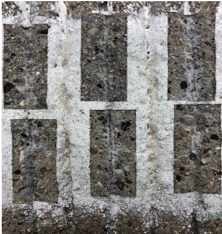
Figure 6: Photograph of a white paint stripe on concrete specimen with different ablated regions.
