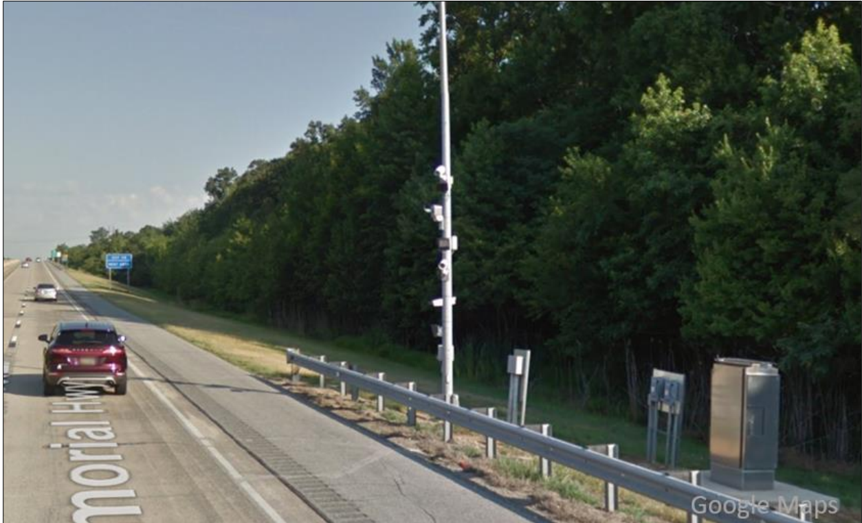
Figure 2. Permanent APRS Installation at the Delaware Site Along DE-1
