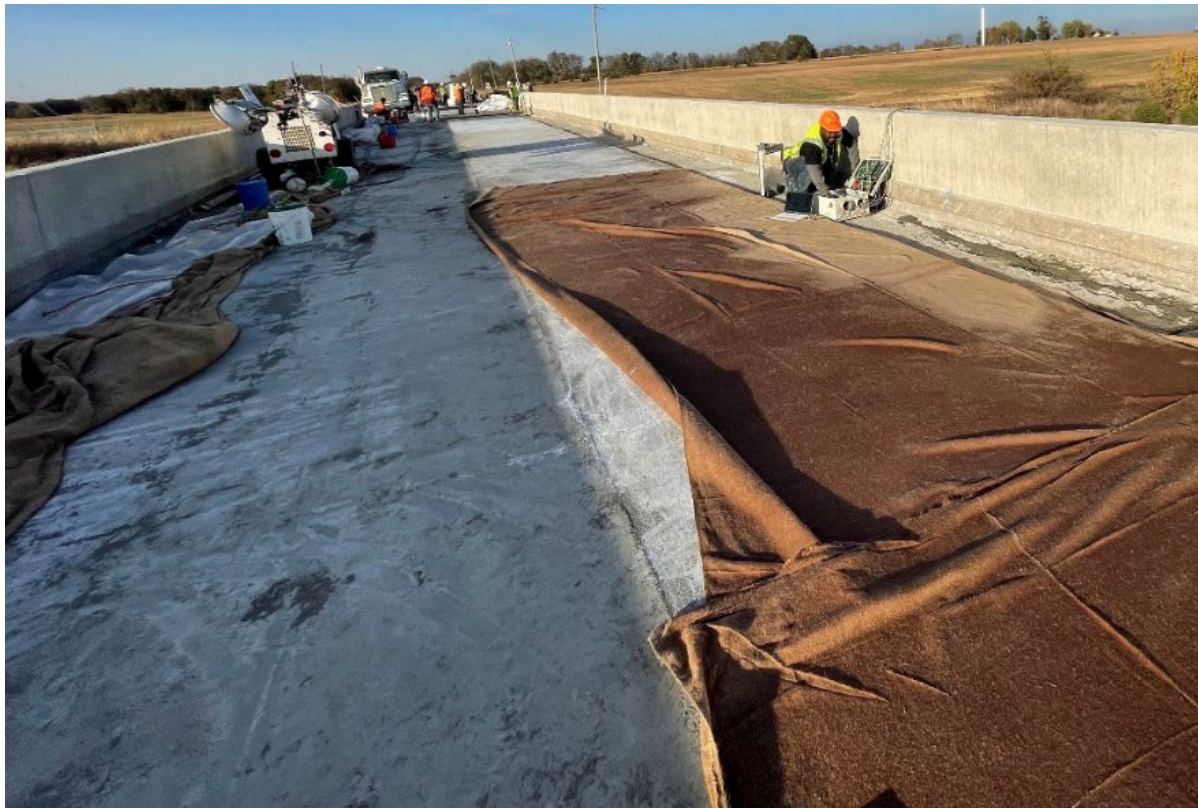
Figure 5.32 North Bound lane overlay surface with improper moist curing 2 d after casting (left) and South bound lane surface shortly after casting with non-uniform moist curing (right)
