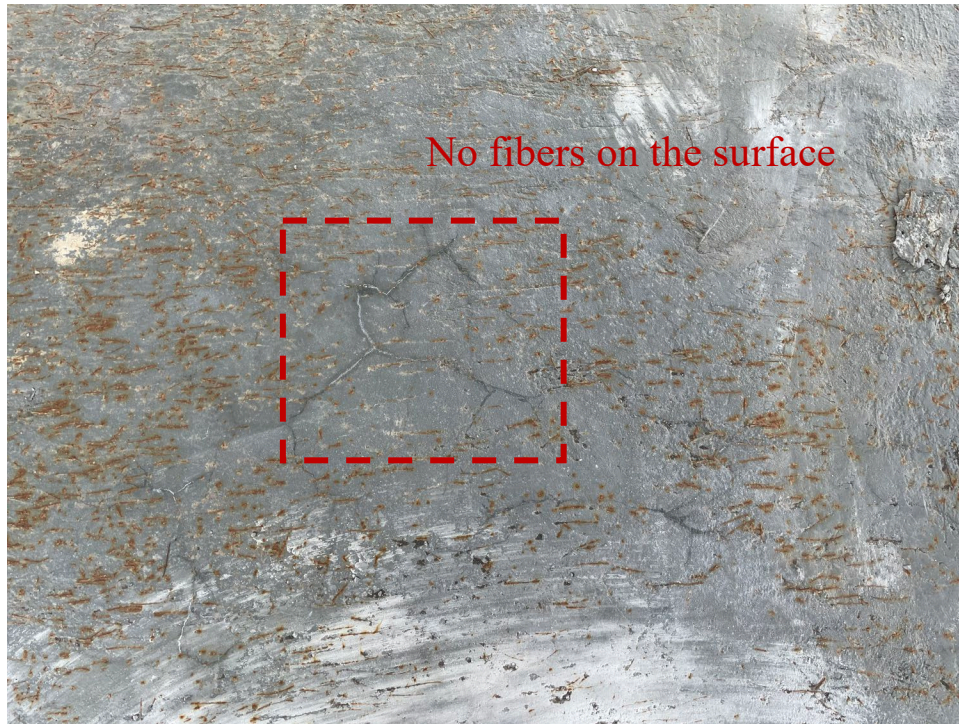
Figure 5.14 Surface of the mockup overlays of (a) mockup A and (b) mockup B after approximately 5 months of outdoor exposure (c) closeup view of cracks on mockup B
