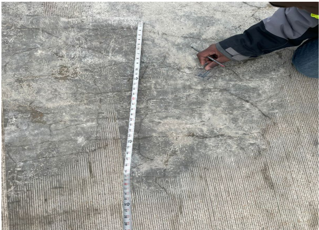
Figure 5.47 Measurement of crack spacing for Route Z Bridge
