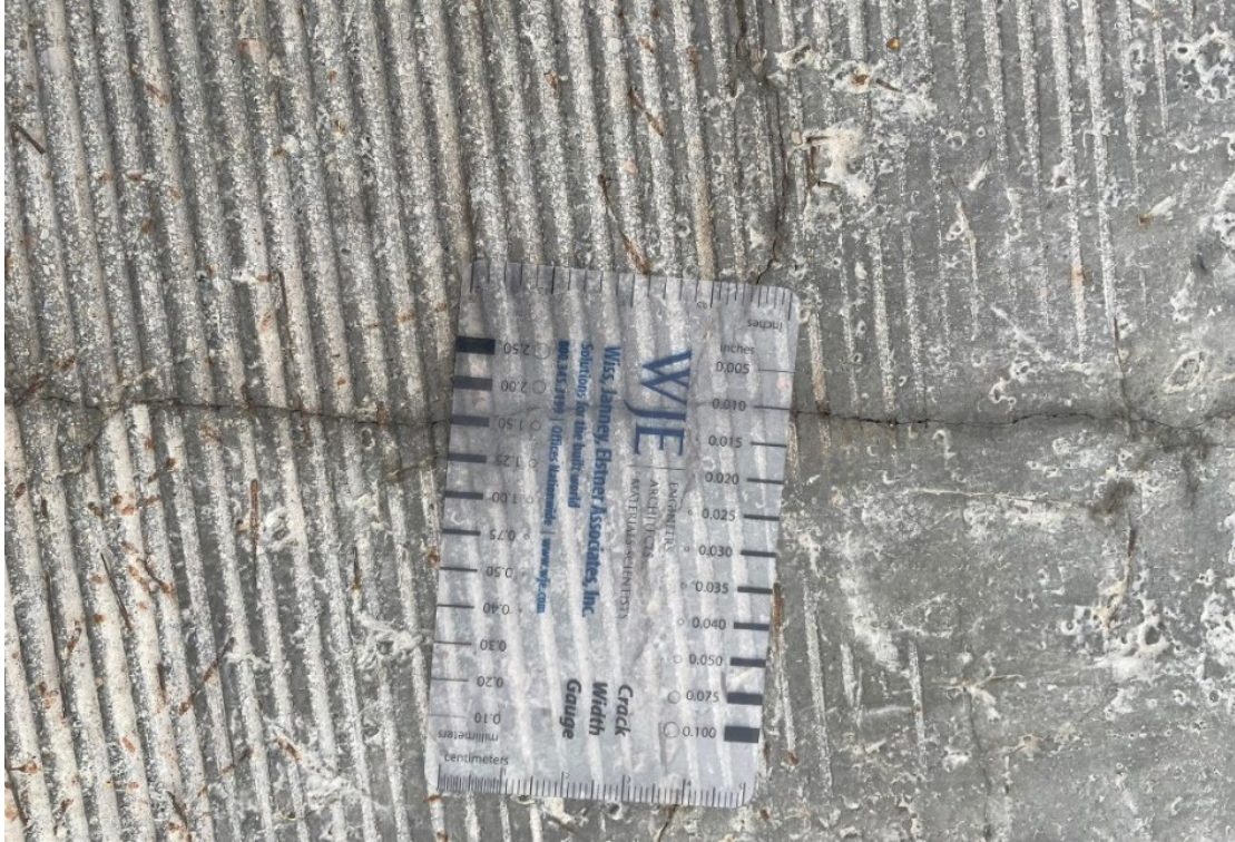
Figure 5.46 Measurement of crack width for Route Z Bridge
