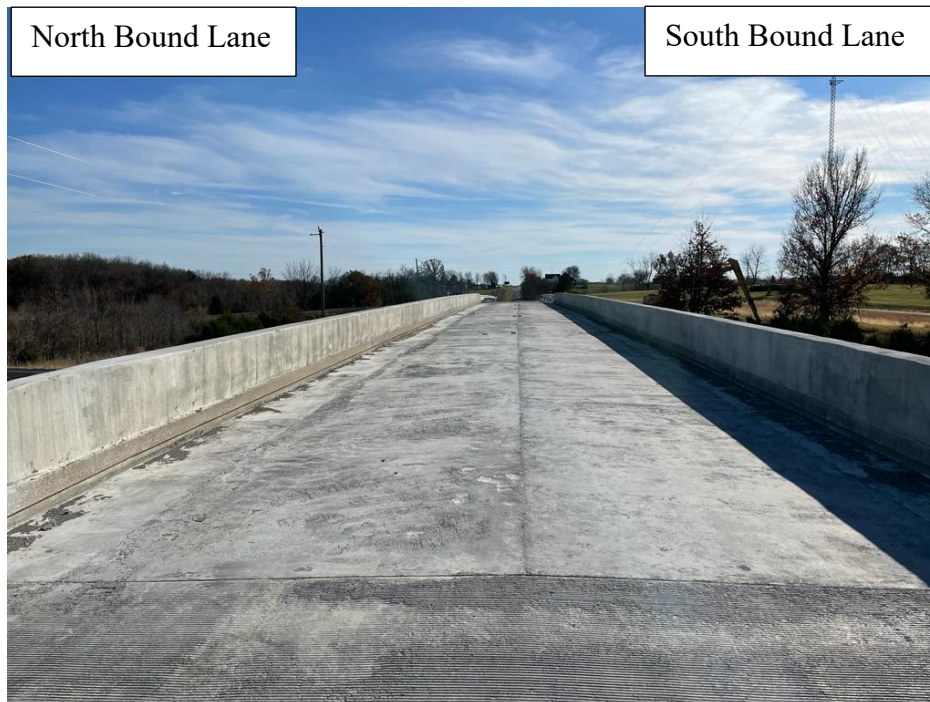
Figure 5.43 Route Z Bridge inspection 7 days after placement indicating no cracking on both North bound and South bound lanes
