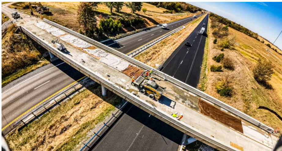
Figure 5.15 Overview of Route Z Bridge with wet burlap to pre-wet subbase before UHPC casting
