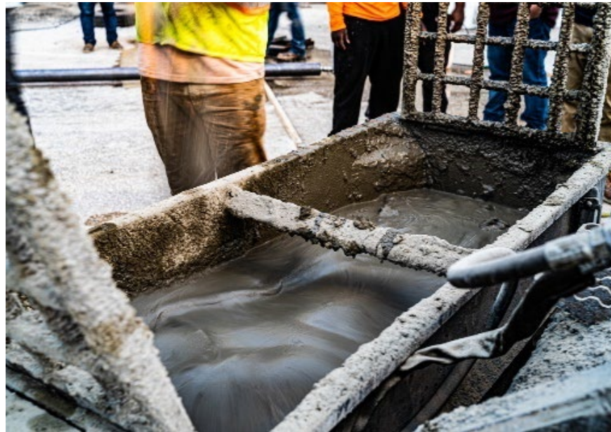
Figure 5.8 Mixing of UHPC using a skid steer concrete mixer (UHPC with excess water used in mockup A)
