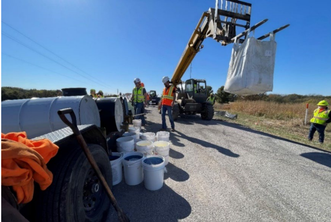
Figure 5.26 Dry materials in supersacs
