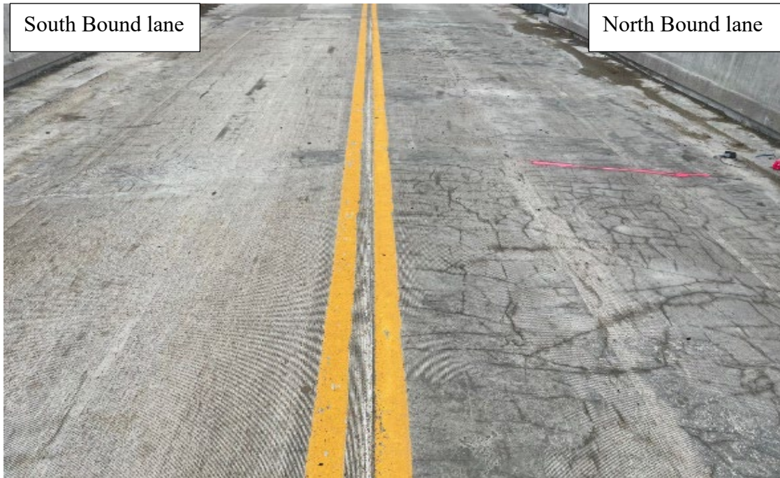
Figure 5.44 Route Z Bridge inspection 96 days after placement showing significant cracking in the North bound lane and no cracking on the South bound lane
