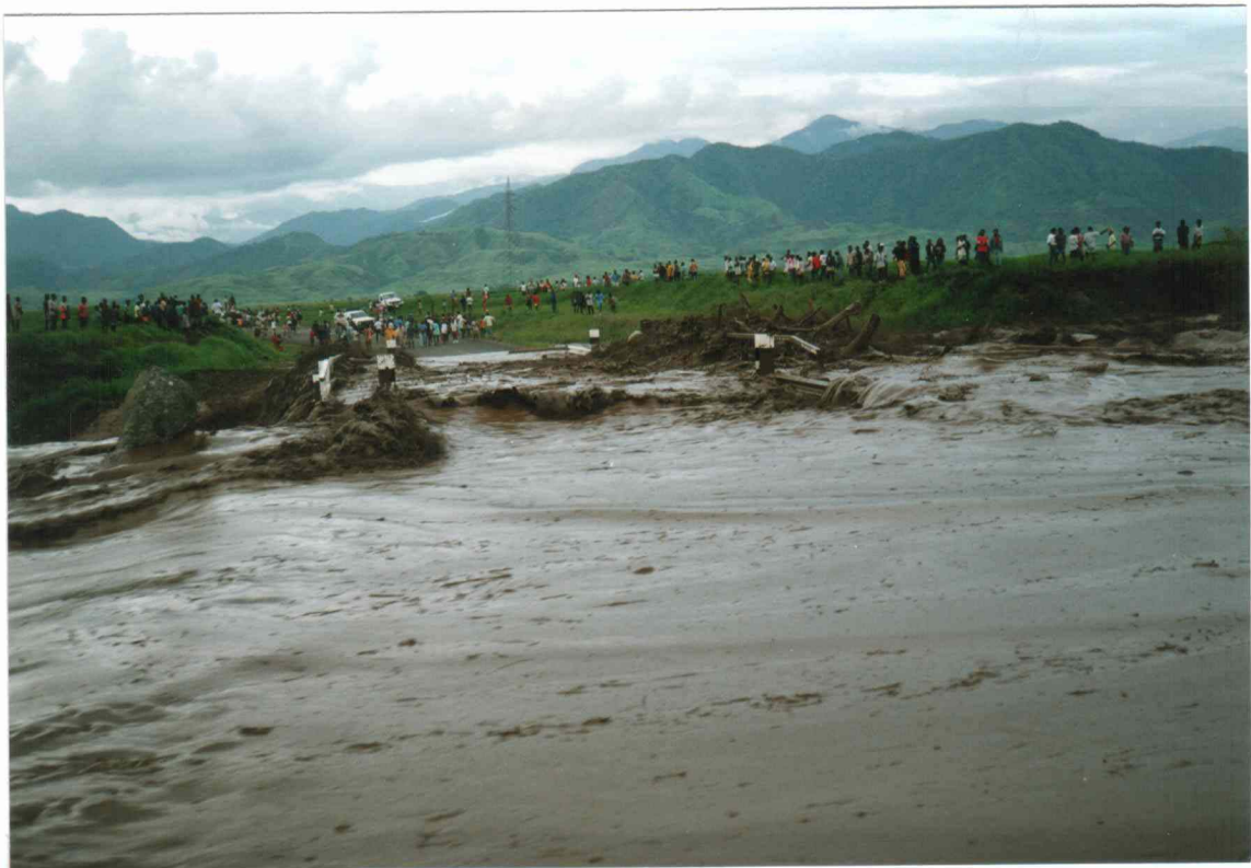
Figure 7.13 Landslide induced flooding overtops and washes away the Bura bridge.
