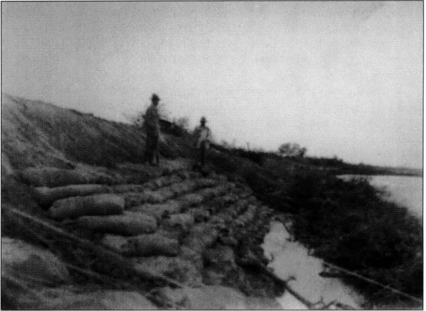
Figure 1. Jorge von Hauenschild (left) and unknown person in the field. Construction of the water management system in Río Dulce. Photo from the collection of photos belonging to the von Hauenschild collection. Image courtesy of the von Hauenschild collection at the Museo de Antropología, FFyH, UNC.
