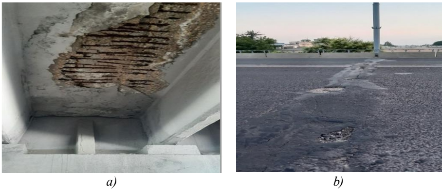
Fig. 2. Defects and damage to bridges and overpasses in Tashkent: a is defects and damage in the lower part of the slab span; b is roadway defects and cracks in the expansion joint constructions
