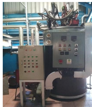
Figure 2. Burner / Thermal Tank
