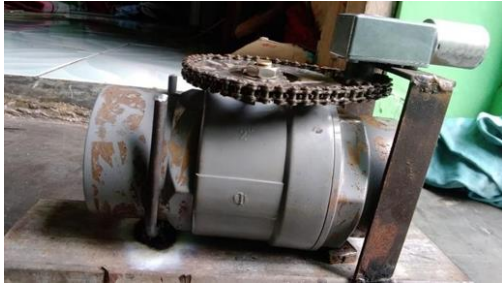
Gambar 8. MOV ( Motor Operated Valve )
