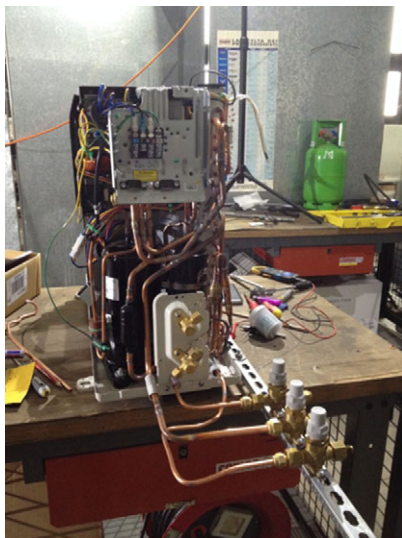
Figure 3. Air-to-air heat pump, as modified.
