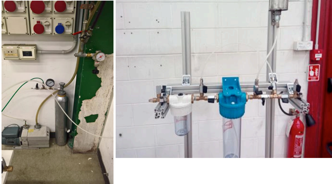
FIG. 8: the low vacuum pump, the vessel for vacuum buffer and the compressed air (left); the oil filling system (right).
