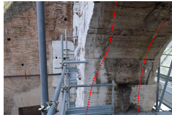
Figure 19. Vertical cracks, highlighted in red, in the internal part of the arch between column 4 and 3.
