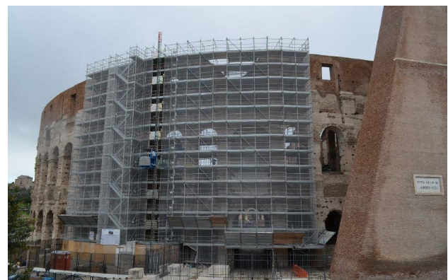
Figure 12. Construction site for the study of the columns affected by the current damage.
