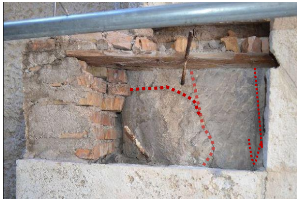
Figure 21. Cracks detected and highlighted in red on the columns of the first floors after removing the travertine slabs in pillar 5.
