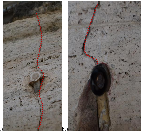
Figure 18. a.) Rebar coming out from the original position, inside of the travertine column and crossed by a sub – vertical crack; b.) Image of the metal bar inside the pillar after removing the cap made by epoxy resin and travertine pieces.
