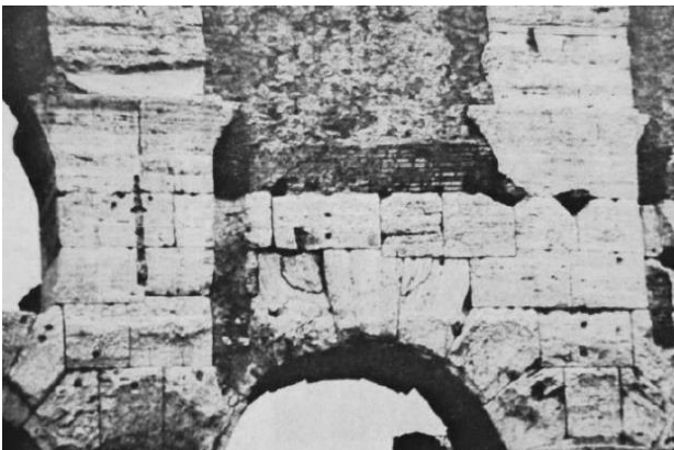
Figure 5. Detail of an arch of the second floor, where the sliding down of the key blocks was observed, as well as different cracks on the travertine blocks.
