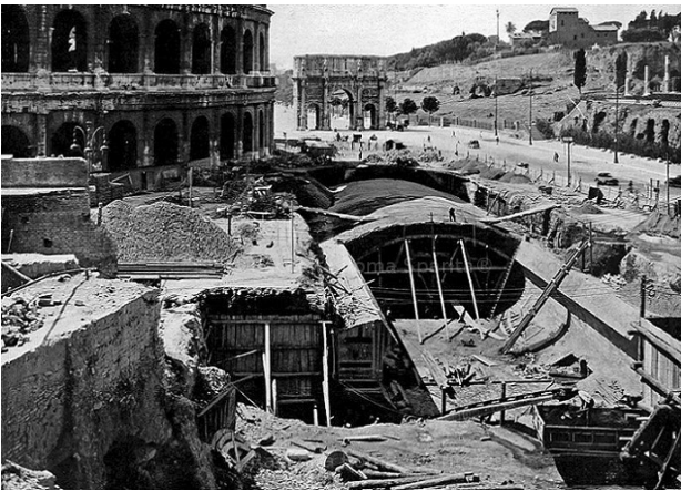
Figure 1. Picture showing the works for the construction of the underground B line around 1940. ( https://www.romasparita.eu/foto-roma-sparita/96998 ).
