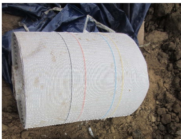
Figure 4: Geotextile strip encasing two single-mode and two multi-mode optical fibres.
