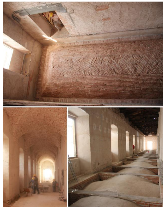
Figure 4. Photo of the restoration of Camponeschi palace realized after the 2009 earthquake: consolidation of the brick vaults with glass fibers.
