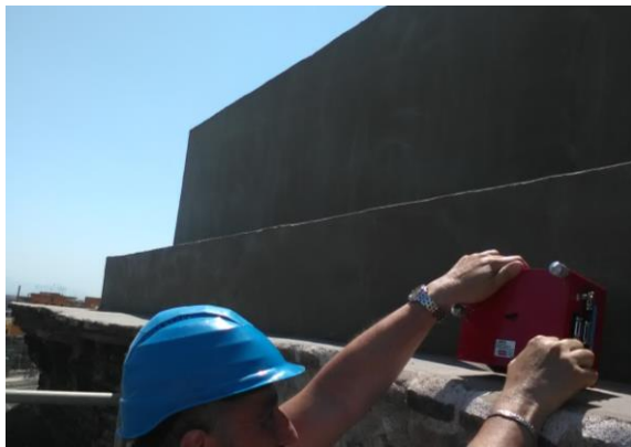
Figure 3. Installation of measurement point A at the dome curb on the north side.
